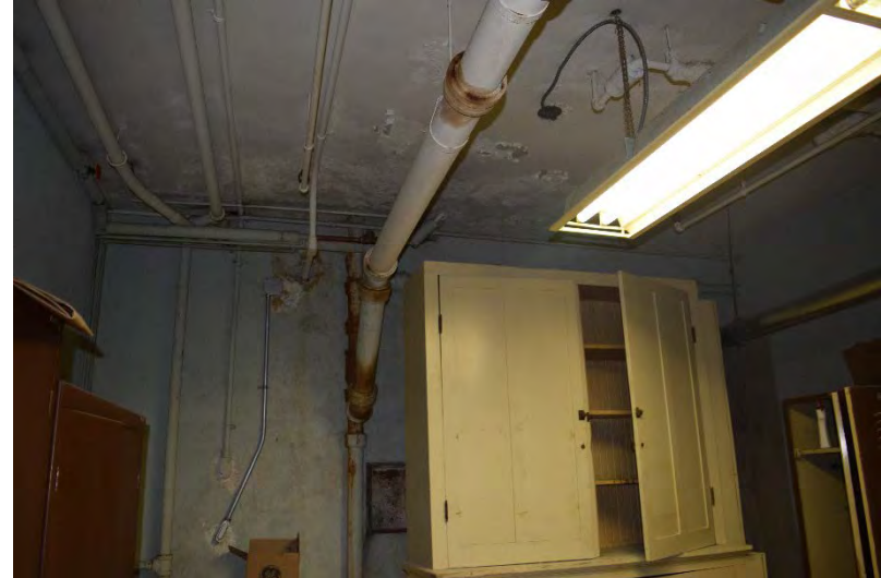
Photo 22: Known asbestos-containing room.
