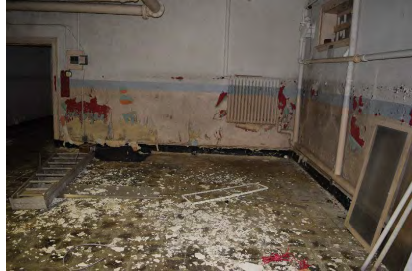
Photo 18: Sprinkler room on first floor.
