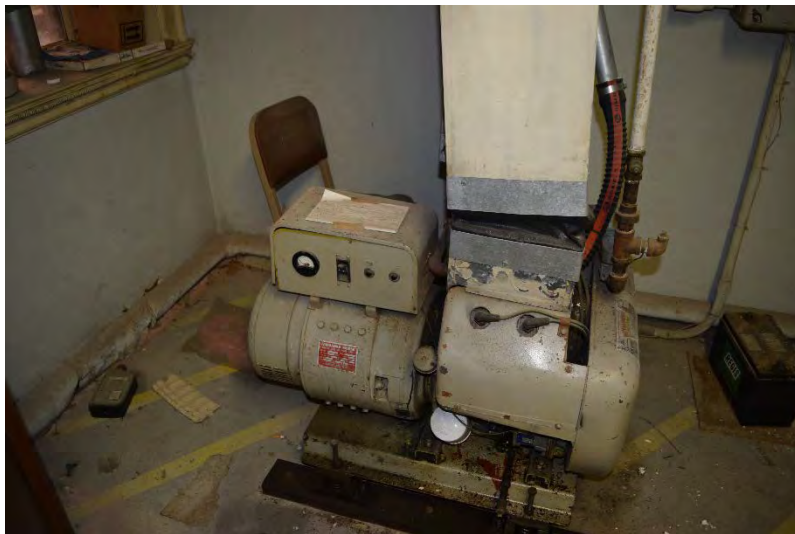
Photo 23: Old generator, not in use.
