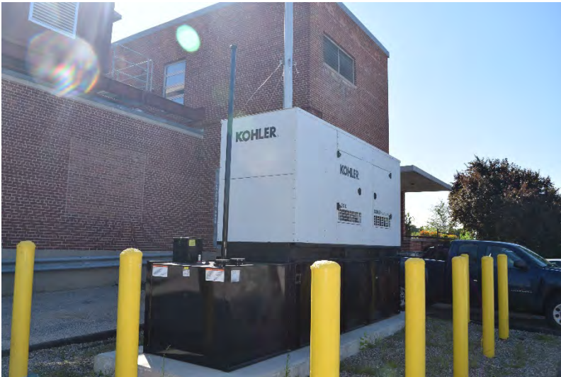
Photo 31: Back-up generator, installed recently.
