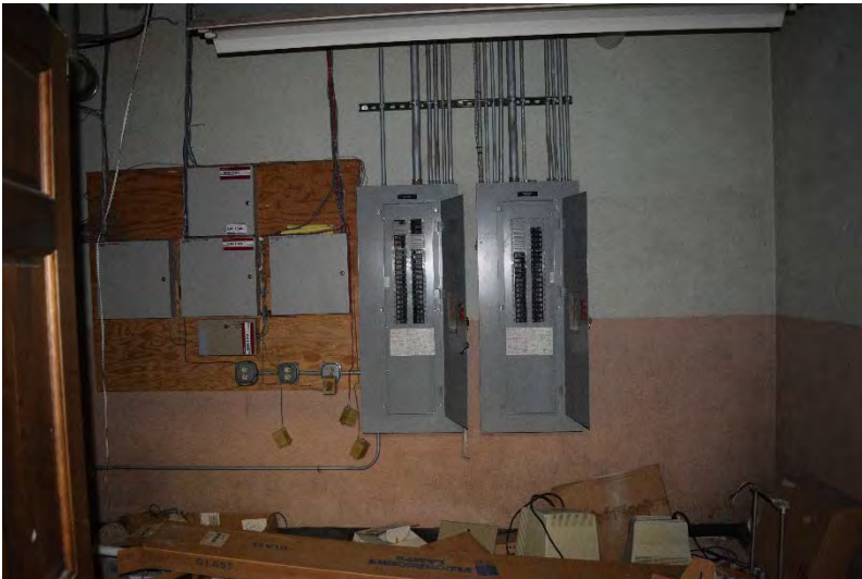
Photo 19: Electric panels on first floor.
