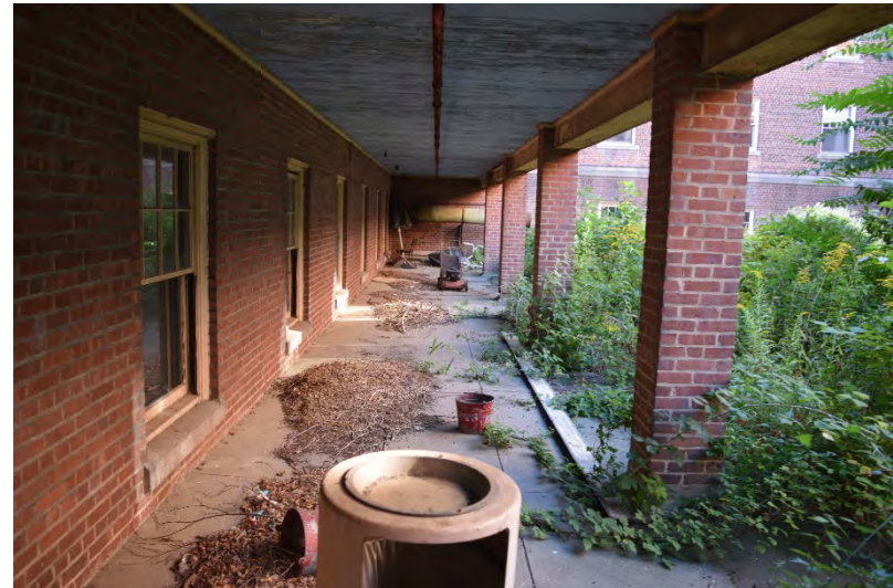
Photo 20: Overgrown courtyard and patio.
