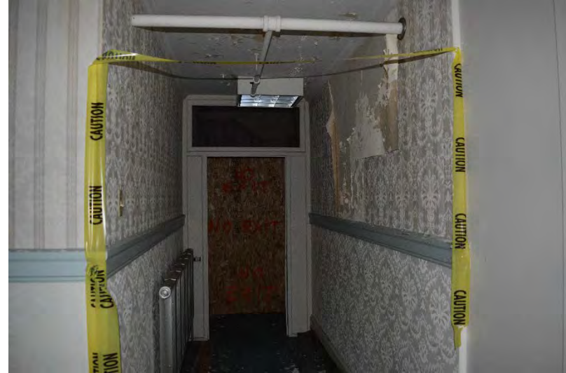
Photo 26: Caution tape and plyboard covering entrance to structurally unstable deck on the second floor.
