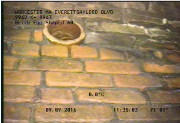
Photo: 9943_9942_26102016_14575959____.jpg 71.08FT, Tap Break-In, at 10 o'clock, -, within 8 inches of joint: NO, 6"
