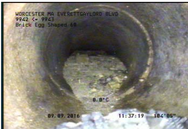
Photo: 9943_9942_26102016_14584646____.jpg 104.38FT, Tap Break-In, at 09 o'clock, -, within 8 inches of joint: NO, 6"
