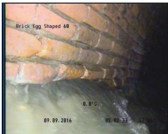
Photo: 12745-9936_09092016_MB_52.3882_080431_A.JPG 52.39FT, Missing Brick, at 08 o'clock
