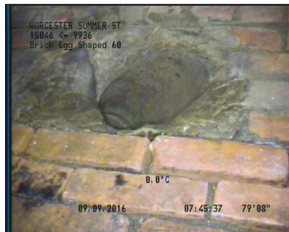
Photo: 9936-15046_09092016_TB_79.6821_074733_A.JPG 79.68FT, Tap Break-In, at 03 o'clock, -, within 8 inches of joint: NO, 6"
