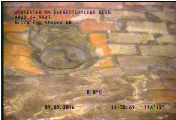
Photo: 9943_9942_26102016_14591818____.jpg 114.97FT, Tap Break-In, at 11 o'clock, -, within 8 inches of joint: NO, 6"
