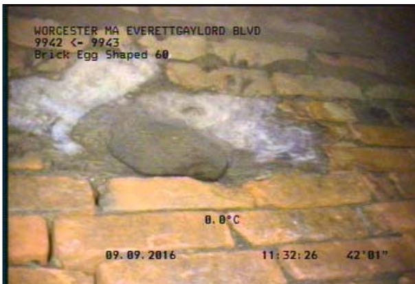
Photo: 9943_9942_26102016_14573434____.jpg 42.09FT, Tap Break-In, at 10 o'clock, -, within 8 inches of joint: NO, 6"
