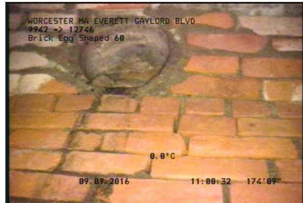
Photo: 9942_12746_26102016_14492020____.jpg 174.76FT, Tap Break-In, at 03 o'clock, -, within 8 inches of joint: NO, 6"
