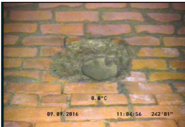
Photo: 9942_12746_26102016_14504242____.jpg 242.05FT, Tap Break-In, at 10 o'clock, -, within 8 inches of joint: NO, 6"
