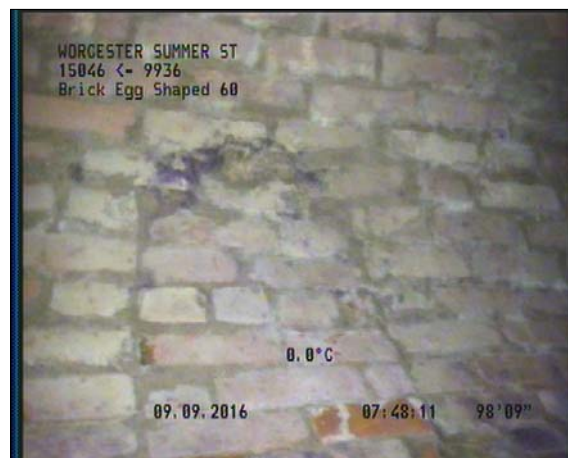
Photo: 9936-15046_09092016_TBC_98.7778_075010_A.JPG 98.78FT, Tap Break-In Capped, at 09 o'clock, -, within 8 inches of joint: NO, 6"
