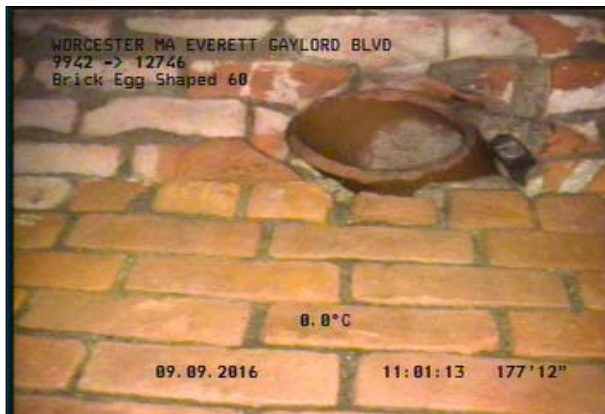
Photo: 9942_12746_26102016_14493939____.jpg 177.96FT, Tap Break-In, at 03 o'clock, -, within 8 inches of joint: NO, 6"
