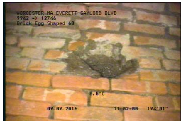
Photo: 9942_12746_26102016_14494646____.jpg 194.16FT, Tap Break-In, at 09 o'clock, -, within 8 inches of joint: NO, 6"
