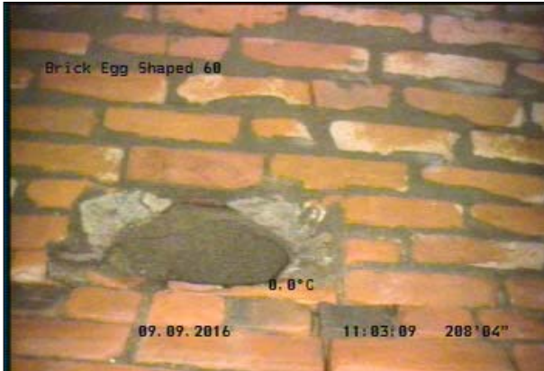
Photo: 9942_12746_26102016_14501818____.jpg 208.35FT, Tap Break-In, at 03 o'clock, -, within 8 inches of joint: NO, 6"
