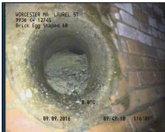
Photo: 12745-9936_09092016_TB_116.7738_095109_A.JPG 116.77FT, Tap Break-In, at 09 o'clock, -, within 8 inches of joint: NO, 6"
