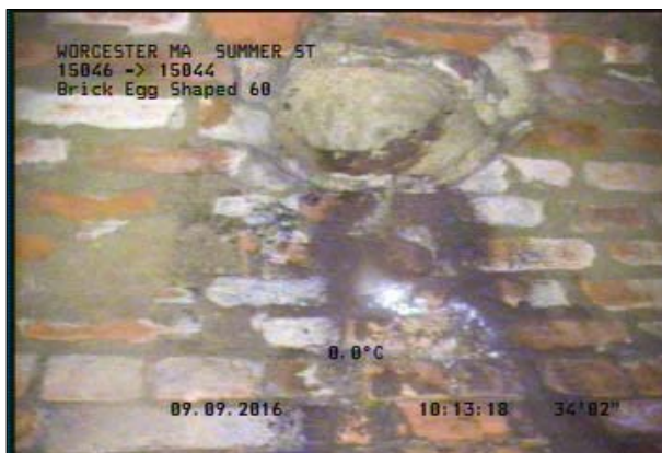
Photo: 15046_15044_26102016_13284848____.jpg 34.19FT, Tap Break-In, at 03 o'clock, -, within 8 inches of joint: NO, 6"
