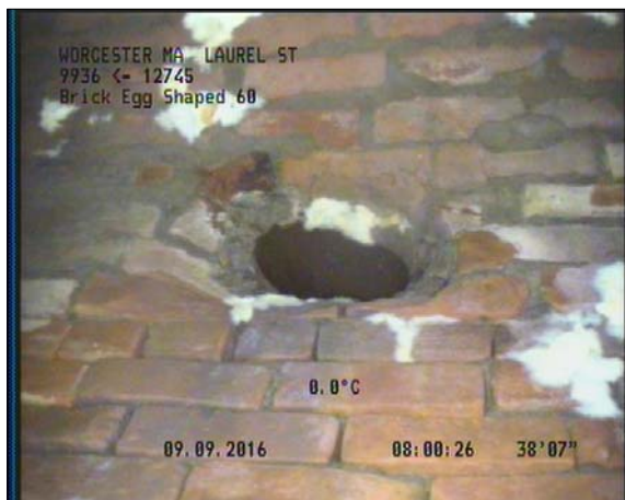
Photo: 12745-9936_09092016_TB_38.5913_080225_A.JPG 38.59FT, Tap Break-In, at 10 o'clock, -, within 8 inches of joint: NO, 6"
