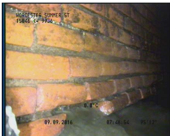
Photo: 9936-15046_09092016_DB_95.9784_074852_A.JPG 95.98FT, Displaced Brick, at 08 o'clock
