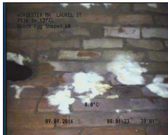
Photo: 12745-9936_09092016_DAGS_39.0912_080321_A.JPG 39.09FT, Deposits Attached Grease, 5 %of cross sectional area, from 09 to 12 o'clock, , within 8 inches of joint: NO
