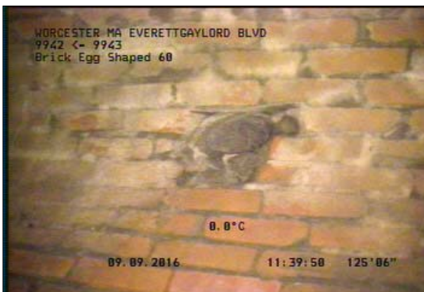
Photo: 9943_9942_26102016_14593434____.jpg 125.47FT, Tap Break-In, at 01 o'clock, -, within 8 inches of joint: NO, 6"
