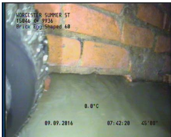
Photo: 9936-15046_09092016_MB_45.6897_074417_A.JPG 45.69FT, Missing Brick, at 08 o'clock
