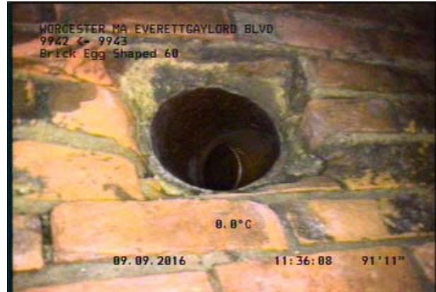
Photo: 9943_9942_26102016_14581818____.jpg 91.88FT, Tap Break-In, at 09 o'clock, -, within 8 inches of joint: NO, 6", 6"
