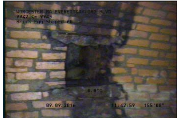
Photo: 9943_9942_26102016_15050707____.jpg 155.66FT, Tap Break-In, at 11 o'clock, -, within 8 inches of joint: NO, 6"
