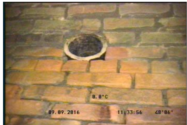
Photo: 9943_9942_26102016_14575050____.jpg 48.49FT, Tap Break-In, at 02 o'clock, -, within 8 inches of joint: NO, 6"
