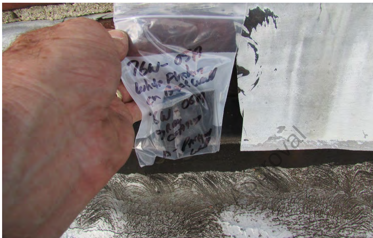
Figure 2 - Tar under White Flashing on Brick
