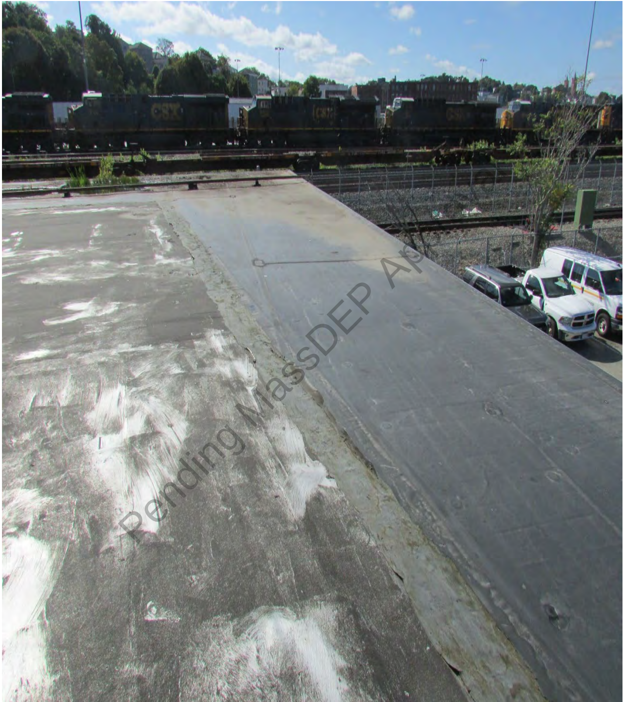
Photo #25 Compromized Roof Area
