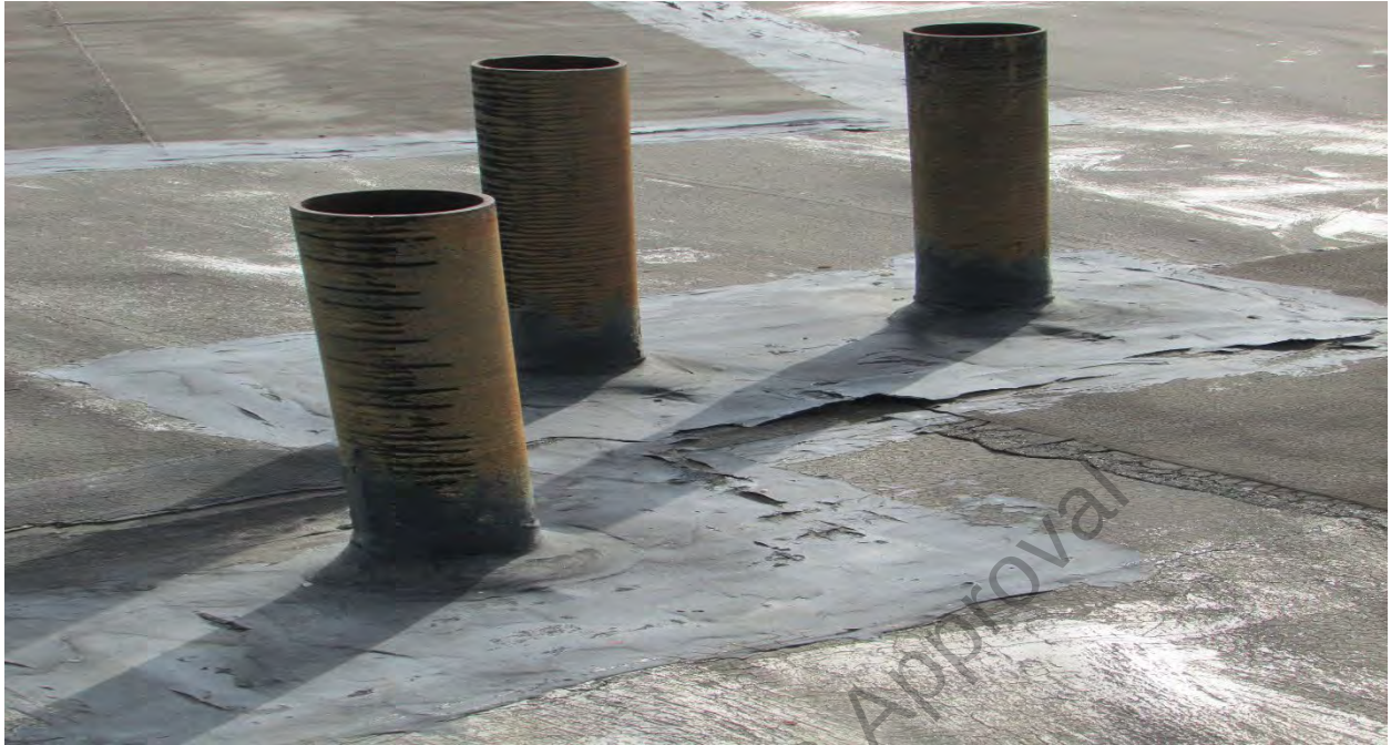
Photo #17 Sample 10A&B Gray Patch Material on Exhaust Pipe (Positive)
