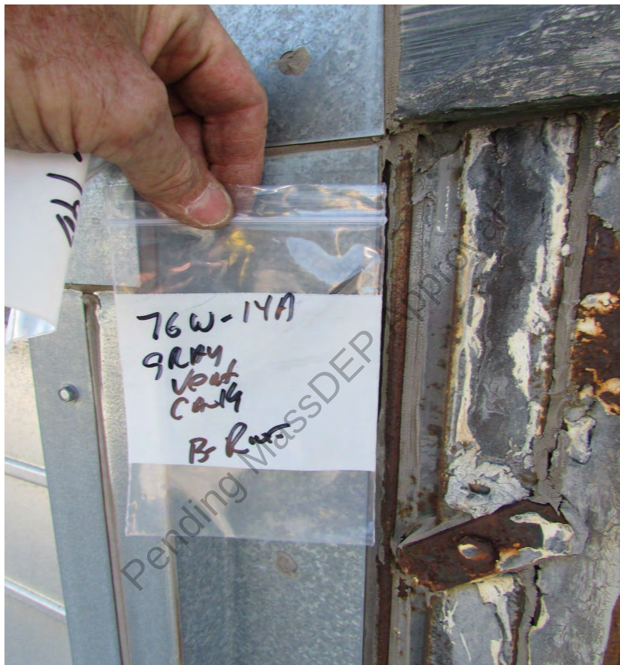
Photo #28 Sample 14A&B Vent Frame Caulk
