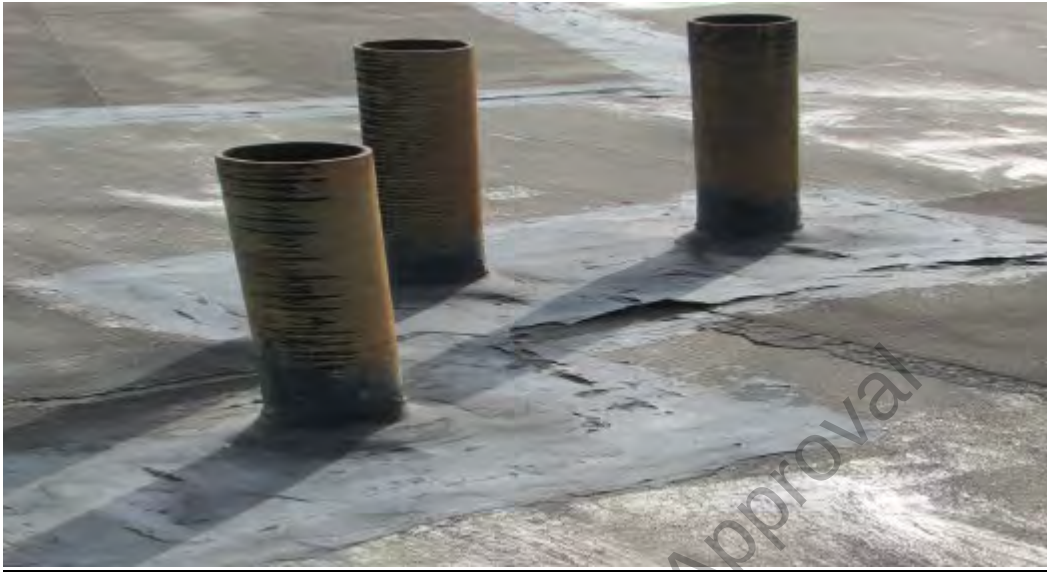
Figure 4 - Gray Patch Material on Exhaust Pipe
