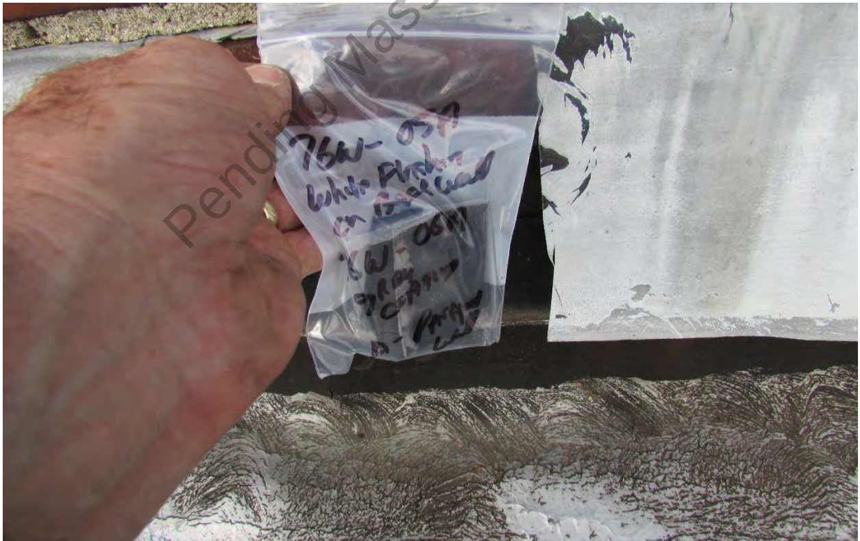
Photo #12 Sample 05/06A&B White Flashing/Tar Under (Positive)
