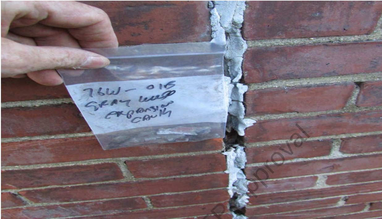
Photo #3 Sample #01A&B Brick Wall Expansion Caulk (Positive)
