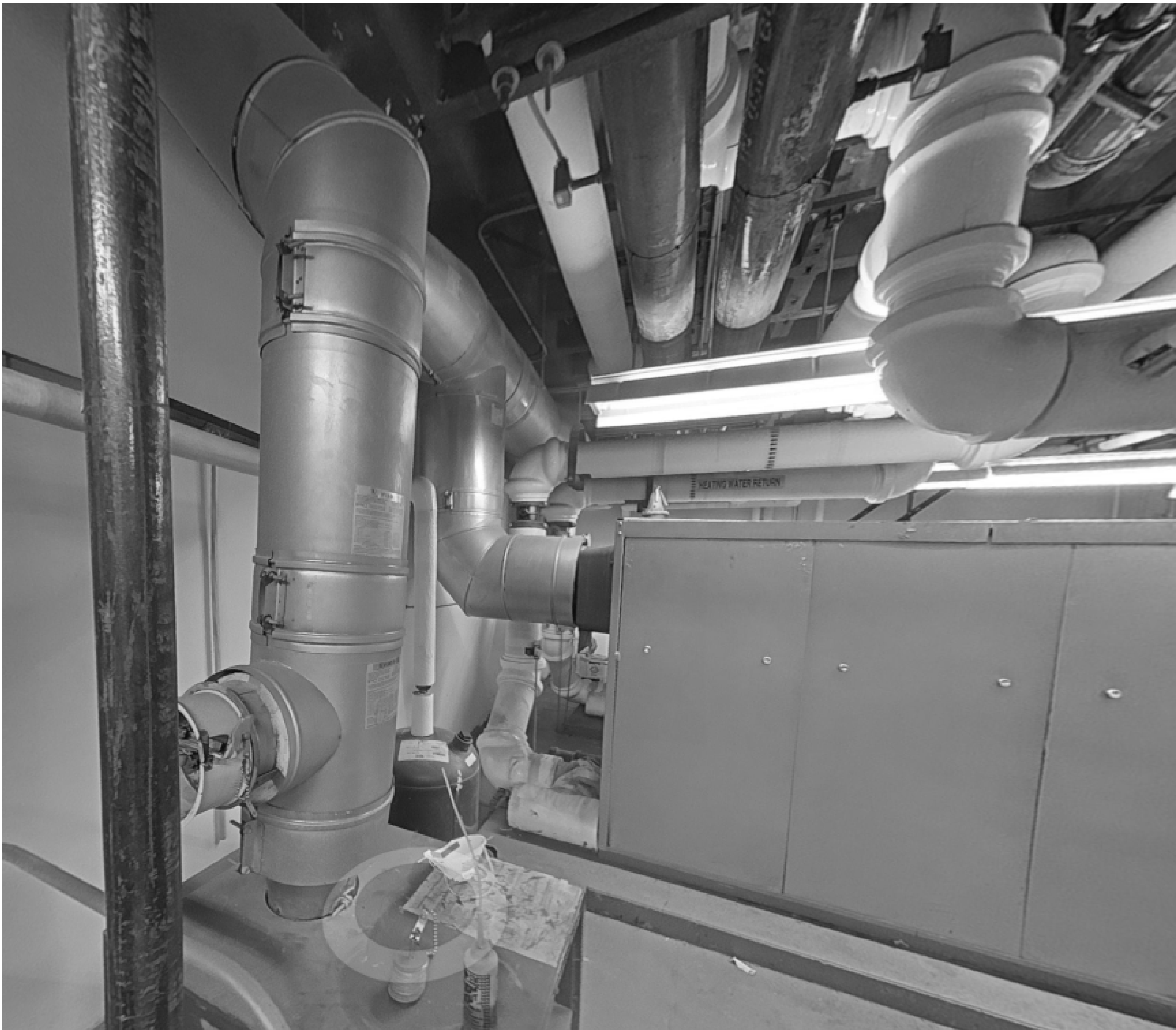
IMAGE 2: EXISTING BOILERS AND WATER HEATER FLUE.
