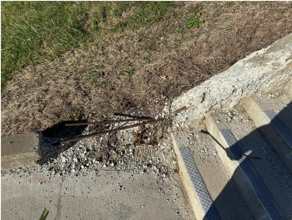
Deterioration of first landing (left)
