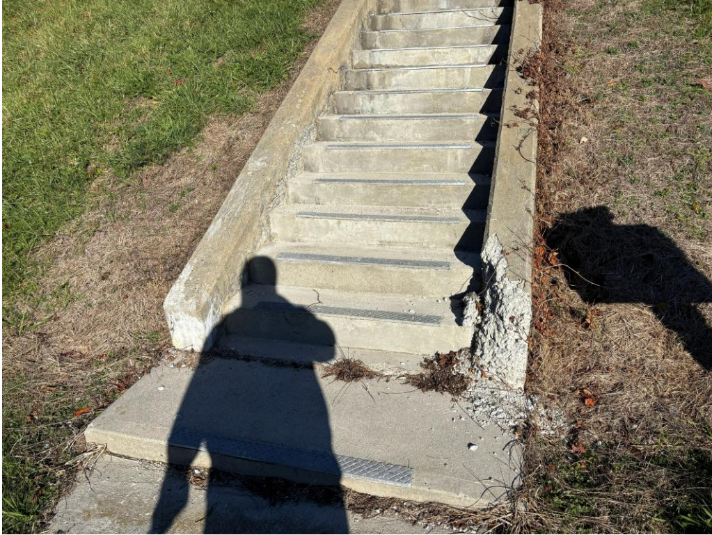
Deterioration at toe of stairs
