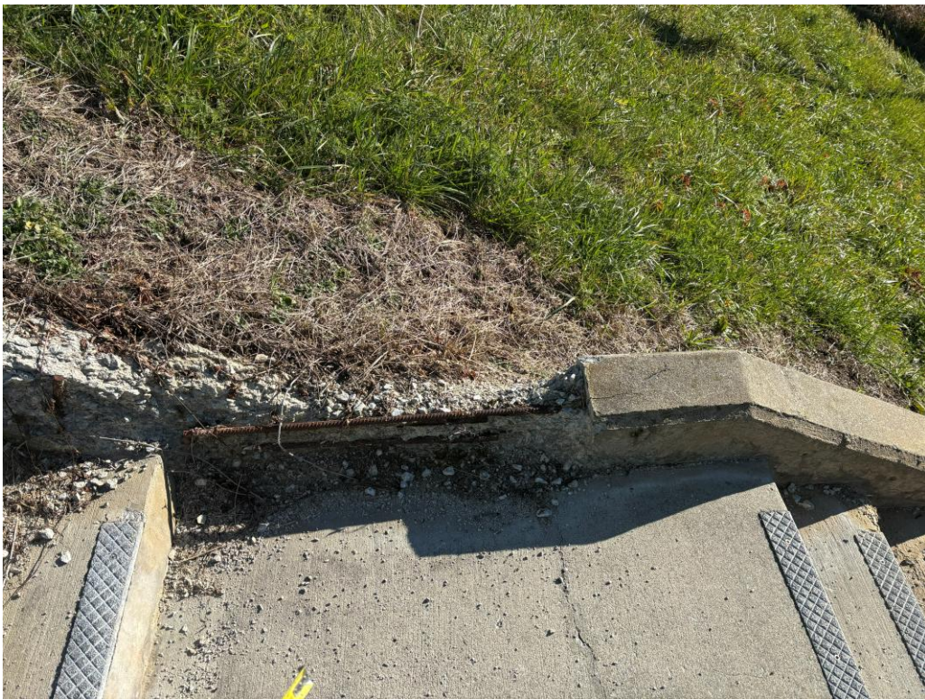
Deterioration at first landing (right)
