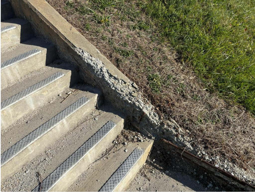
Deterioration at first landing (right)
