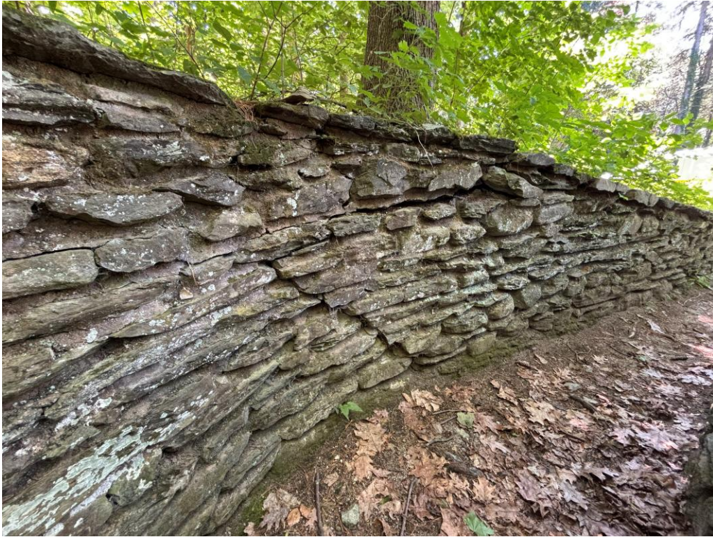
Cracking along right-hand retaining wall
