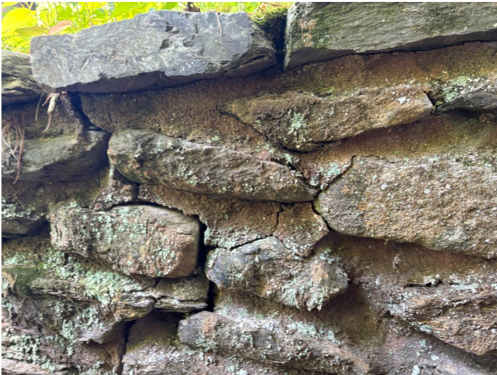
Cracking along left-hand wall
