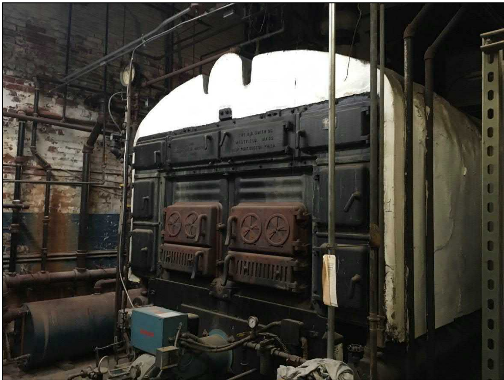
One of two steam boilers on-site; boiler jacket 40% asbestos
