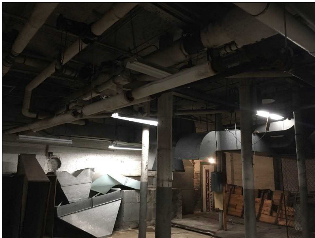
TSI along ceiling; 35-70% asbestos
