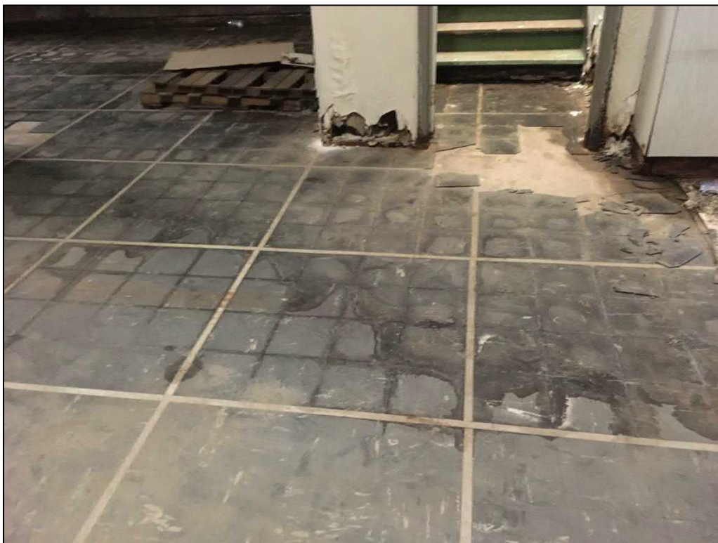
Black 9"x9" floor tiles in basement; 3% asbestos
