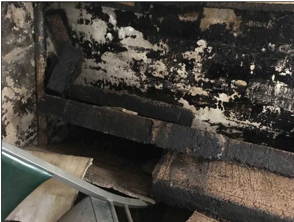
Black coating on cork wallboard, second floor storage room; PCBs 64.4 mg/kg
