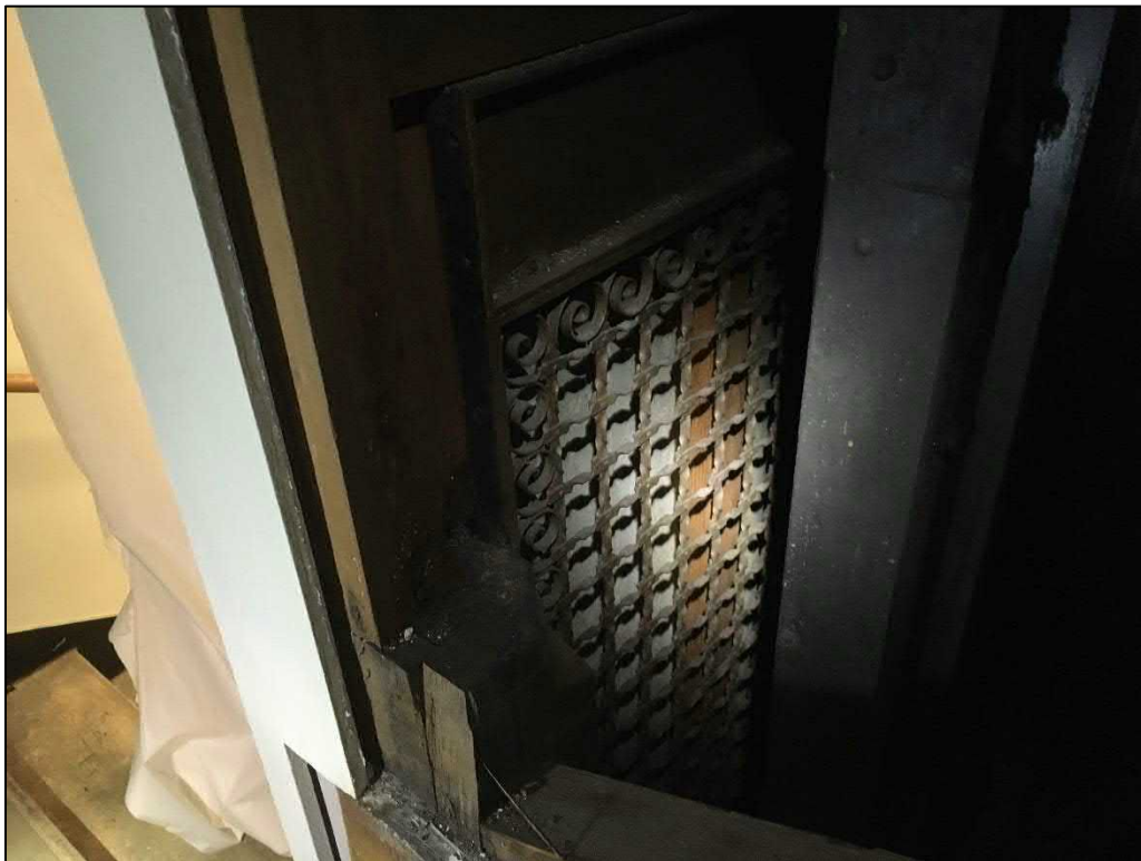
Possible transite panel in freight elevator shaft
