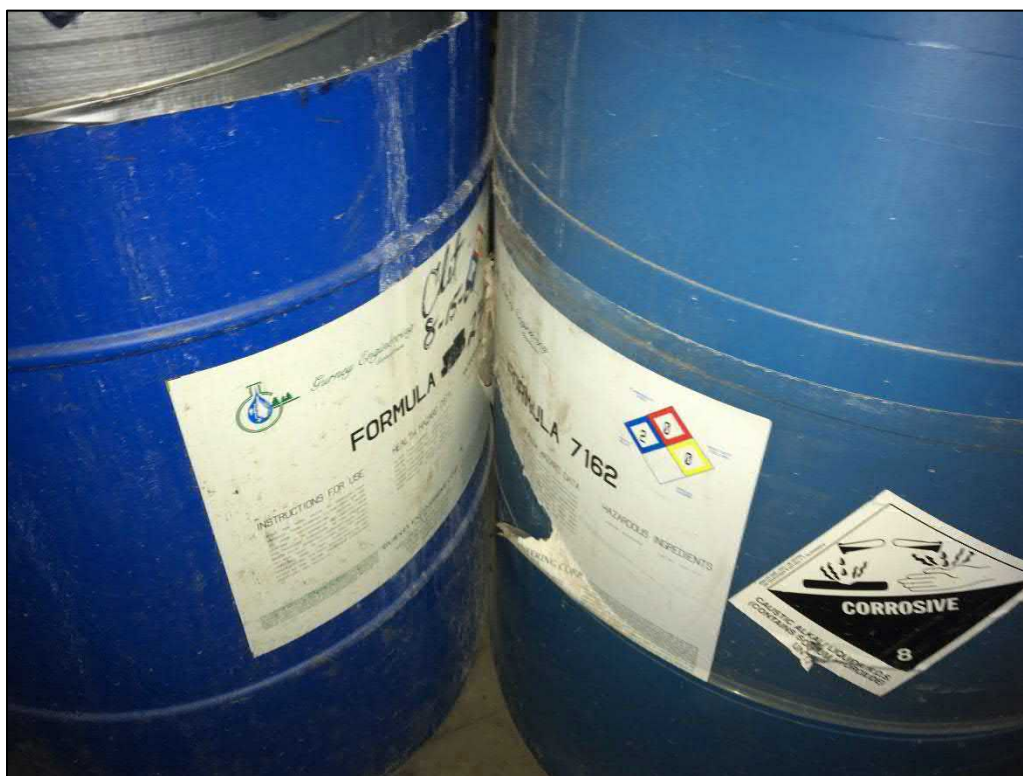
OHMs in boiler room
