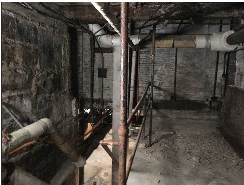
TSI on piping at ceiling and along walls; 35-70% asbestos
