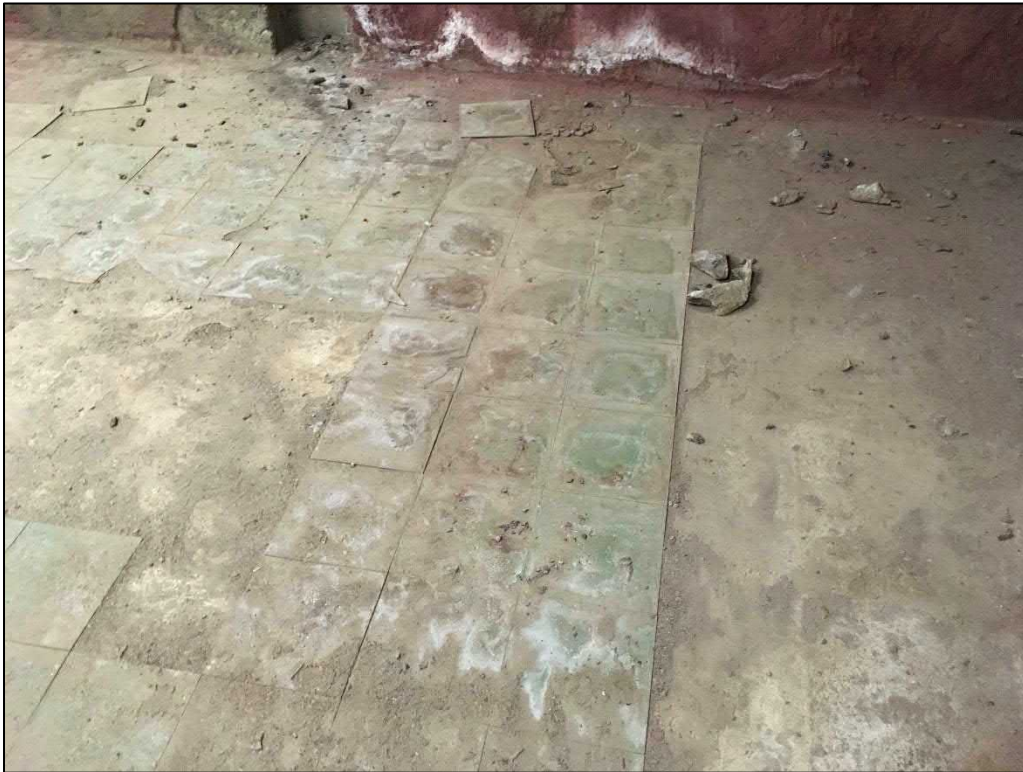
Green 9"x9" floor tiles in basement; 3% asbestos
