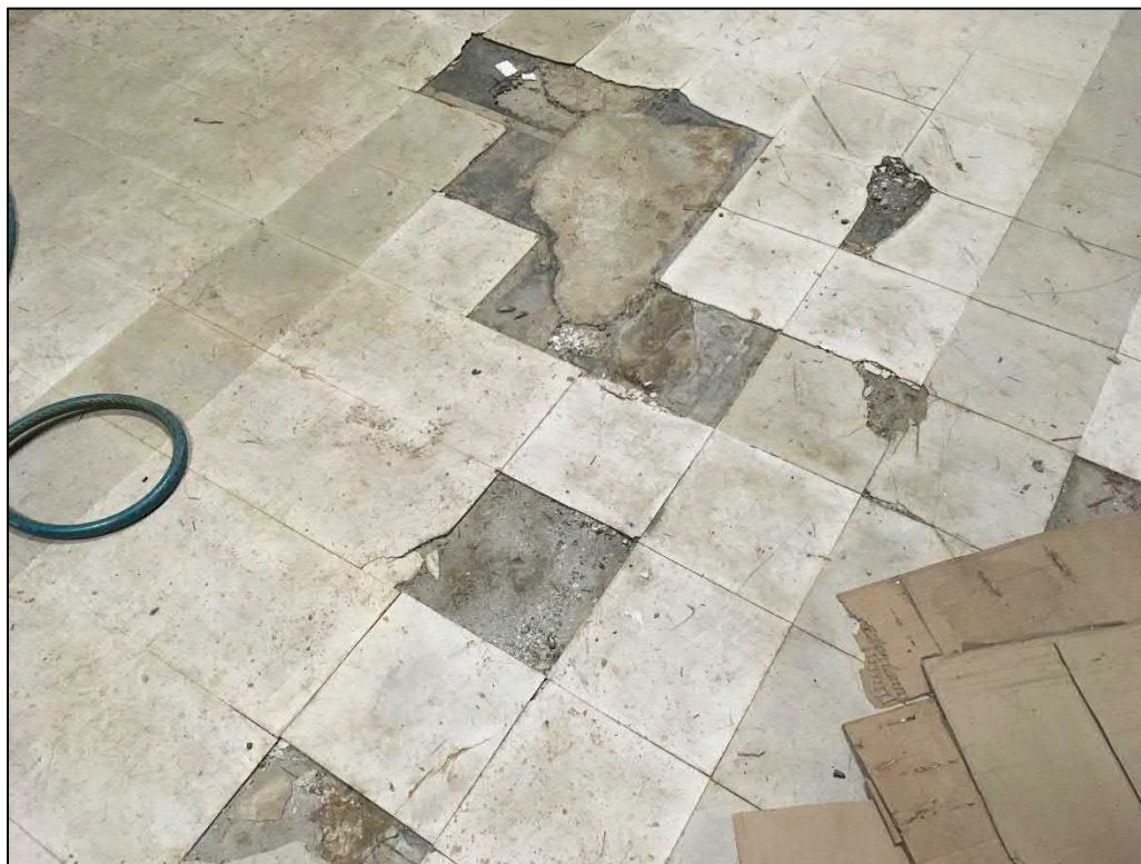
Beige 12"x12" tiles w. mastic (8% asbestos) over black 9"x9" tiles (3% asbestos) over gray leveler (10% asbestos)
