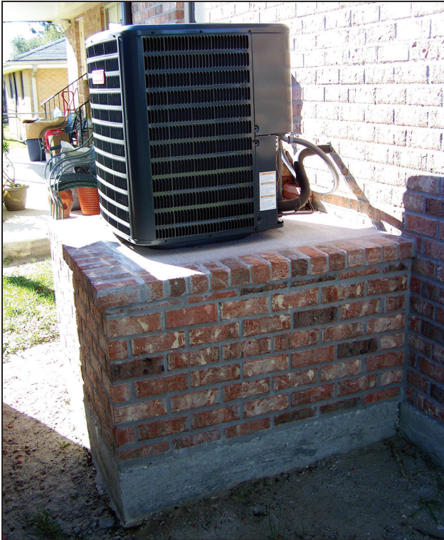
Figure 3-1. Air conditioning compressor elevated on a pedestal.
