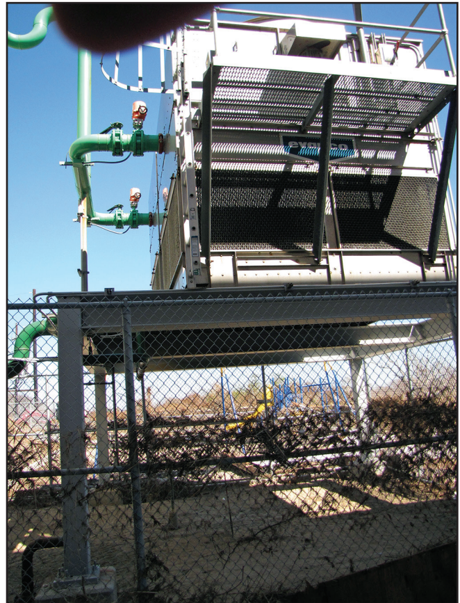
Figure 5-7. Cooling tower placed on an elevated frame (Hurricane Ike, Port Bolivar, Texas, October 18, 2008).
