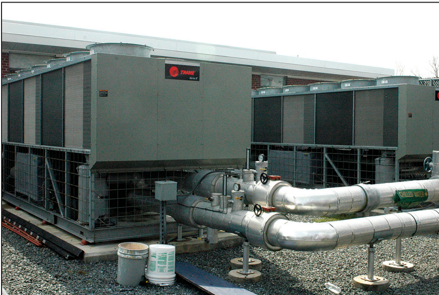
Figure 5-3. Air-Cooled rooftop chiller in Georgetown, Delaware.
