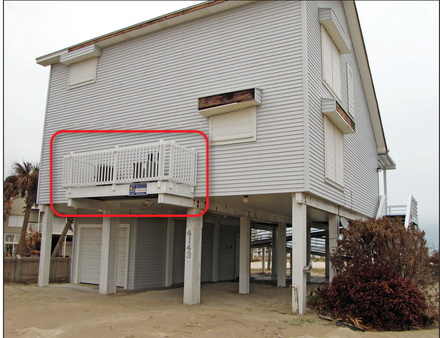
Figure 4-2. Elevated HVAC condenser units in a coastal zone with a protective railing installed (Galveston Island, Texas).
