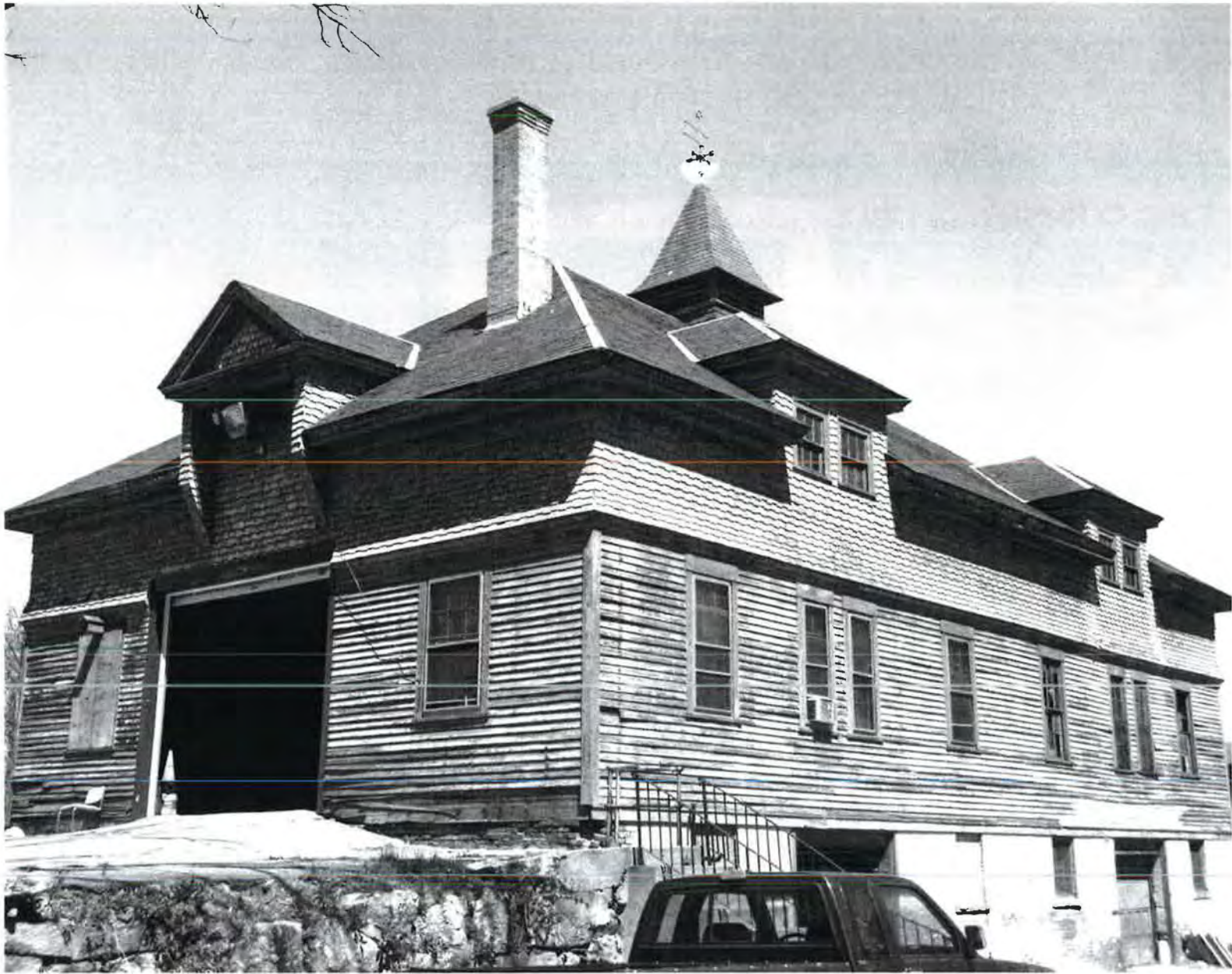
14. Stick style cemetery barn/garage (1889), northwest corner of the cemetery, south facade and east elevation. Looking north. (Photograph: Monique B. Lehner, May 1995)
