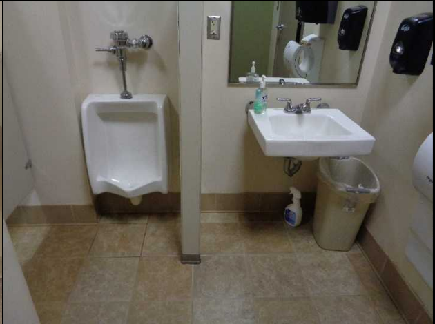
Typical Urinal and Sink
