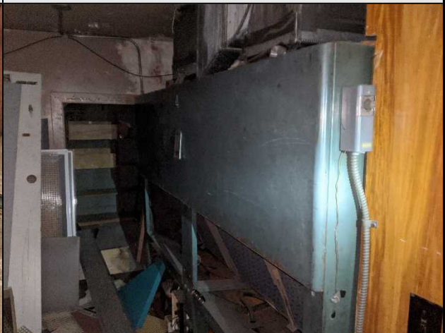
Inoperable Air Handler Unit
