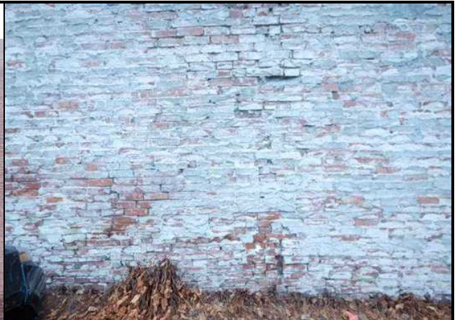
Brick mortar deterioration at southern mural facade
