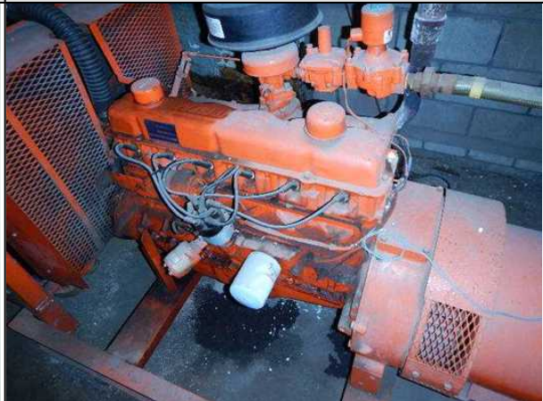
Basement mounted backup generator
