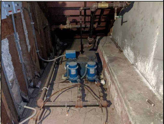
Steam System Piping
