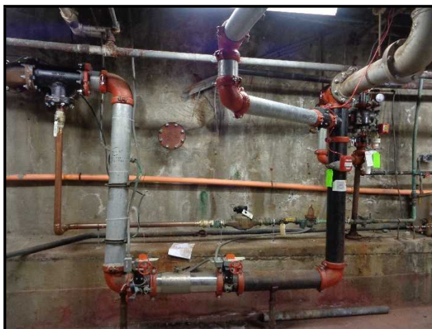
Wet Sprinkler System - North
