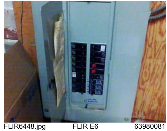
Distribution Panel - No Tag (4th Floor)
