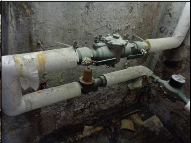
Pipe Insulation and Backflow Preventer
