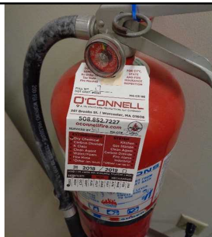
Expired Fire Extinguisher Inspection
