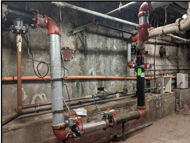
Sprinkler System Piping
