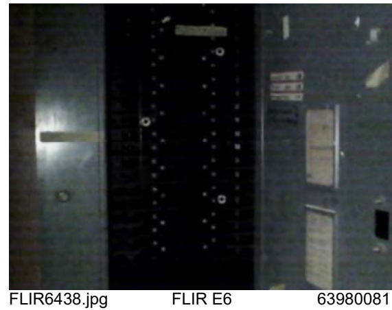
Distribution Panel - 3rd Fl. Annex North. section 2
