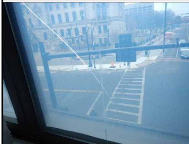
Cracked pane along eastern side of building
