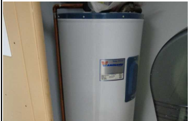
Common Bathroom Water Heater
