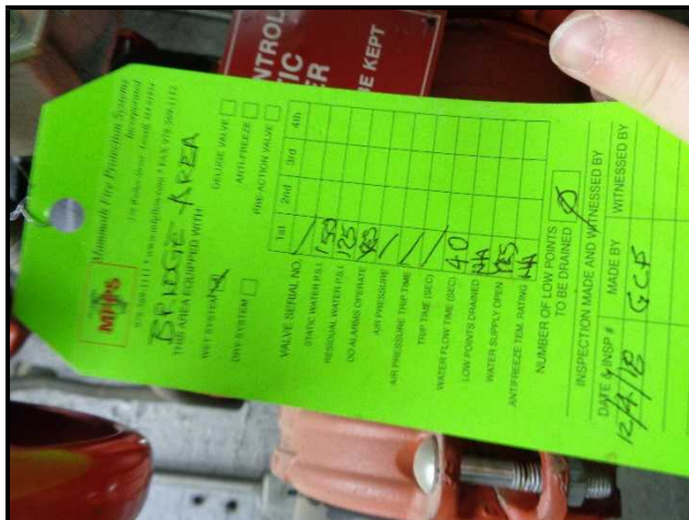
Expired Wet Sprinkler System Inspection
