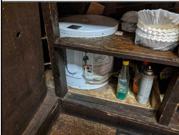
Water Heater Lacking Catch Pan
