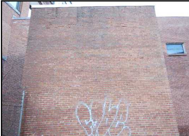
Northern façade brick mortar joint deterioration
