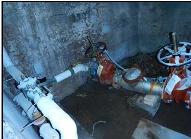
Rear domestic and sprinkler water service line
