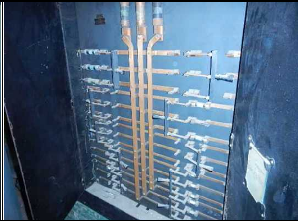
Vintage electrical knife switch panel
