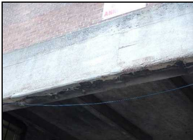
Bottom beam at alleyway bridge southern side showing minor cracking
