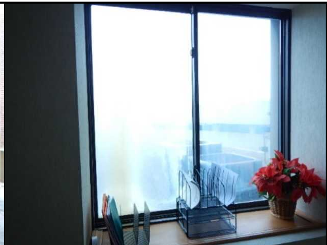
Fogged window pane in office space
