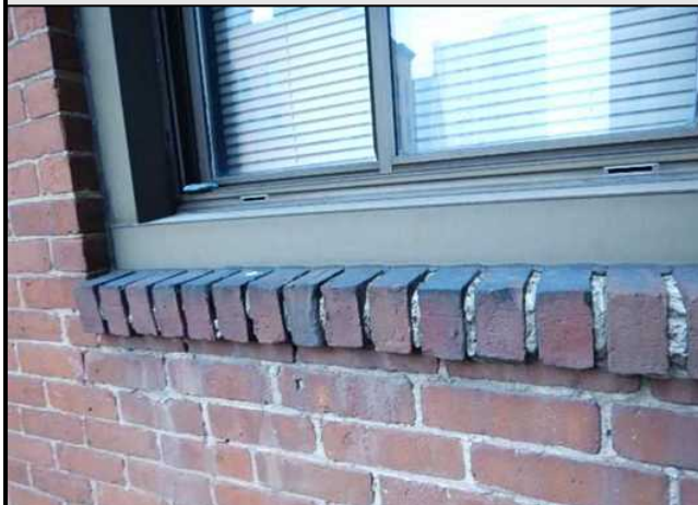
Washed out mortar joints at window sill along northern side
