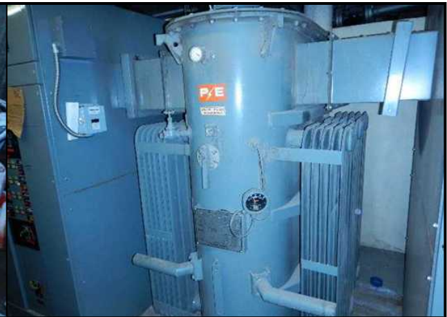
One of two main transformers
