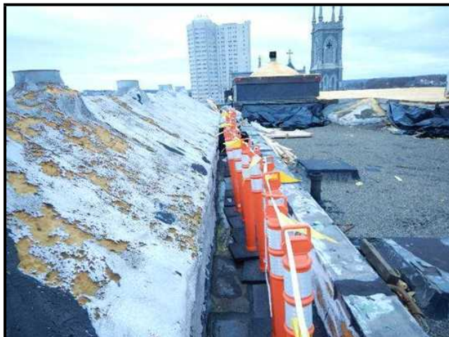
Polyurethane foam roofing showing erosion
