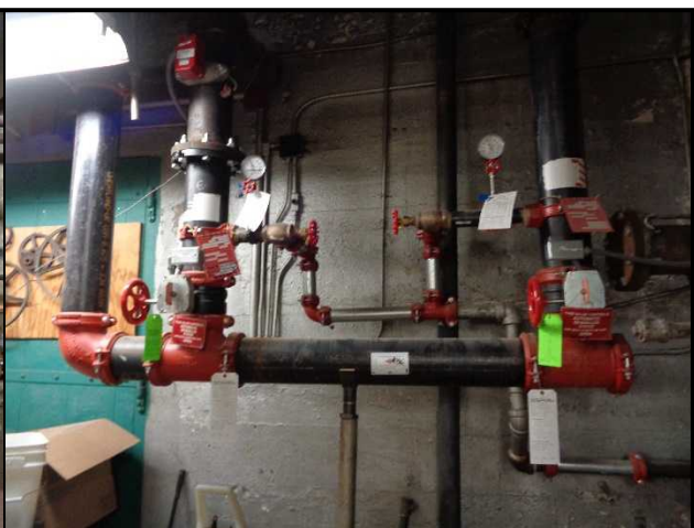
Wet Sprinkler System - South
