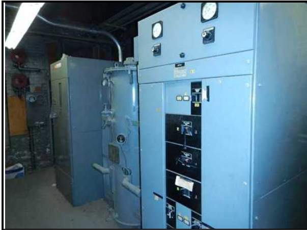
One of two main electrical services
