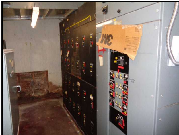
Main Electrical Panels
