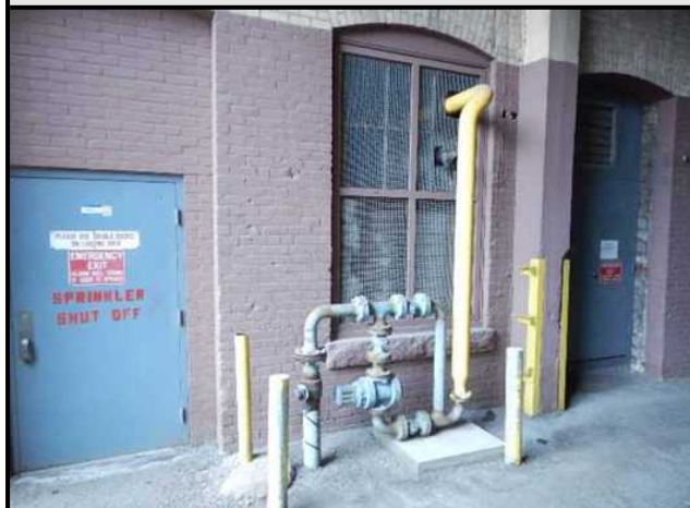
Main gas meter within service alley
