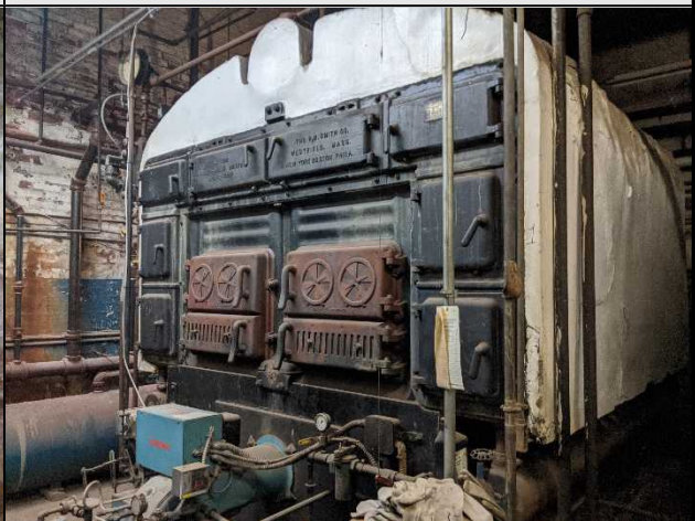
Inoperable Oil-fired boiler
