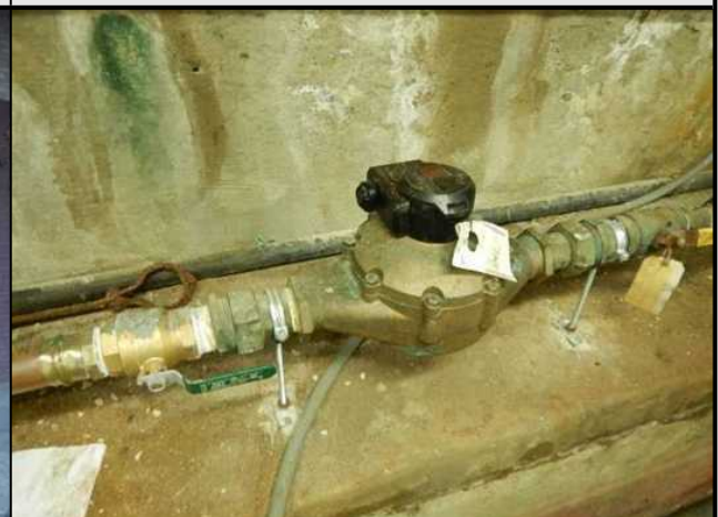
Front of building domestic water meter
