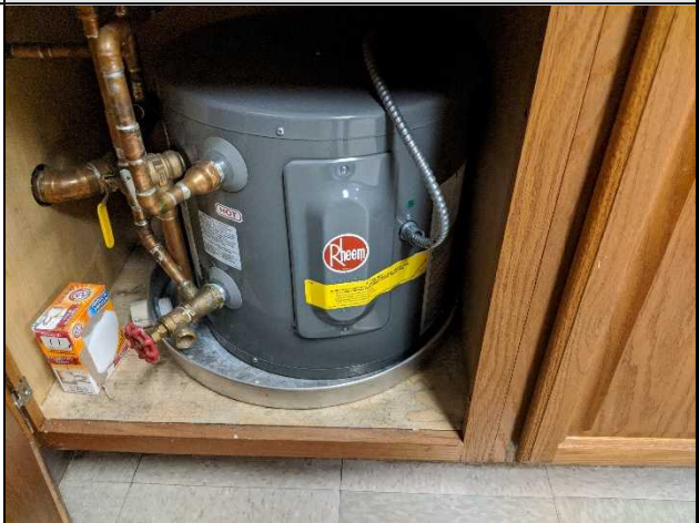
Typical Tenant Space Water Heater
