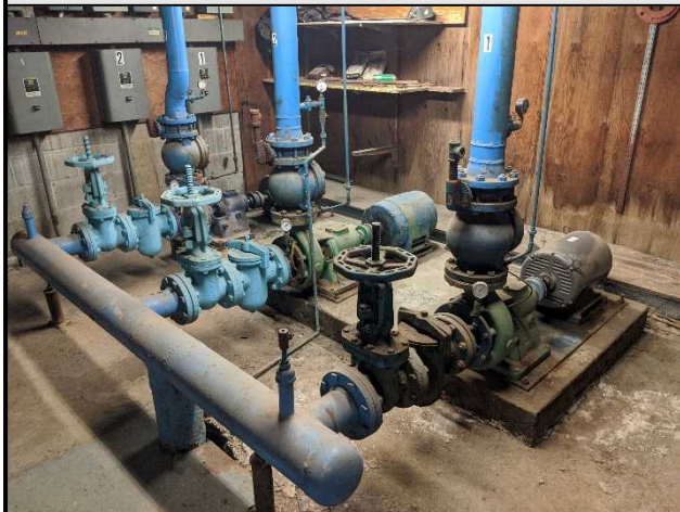
Condenser System Pumps
