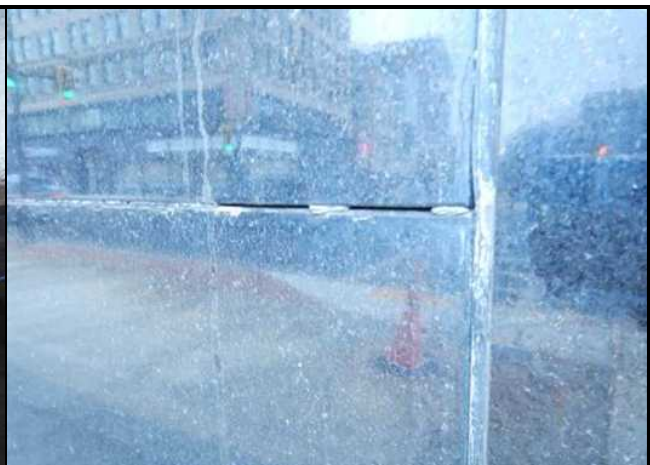
Missing mortar at front of building granite cladding
