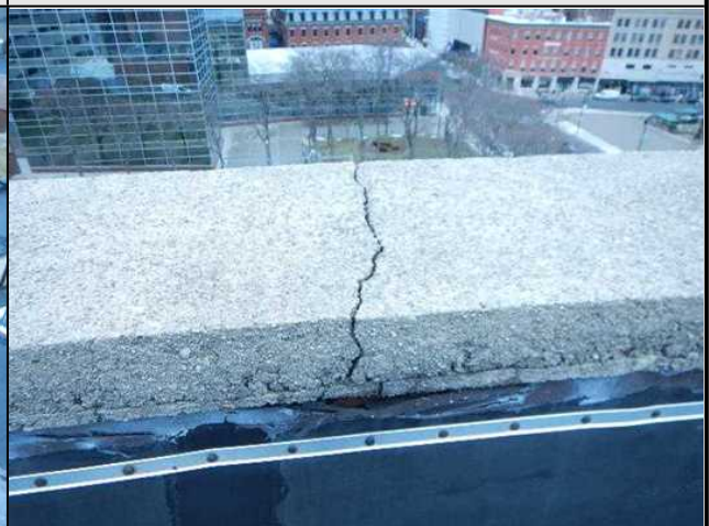
Roof section A/B parapet wall cracked coping
