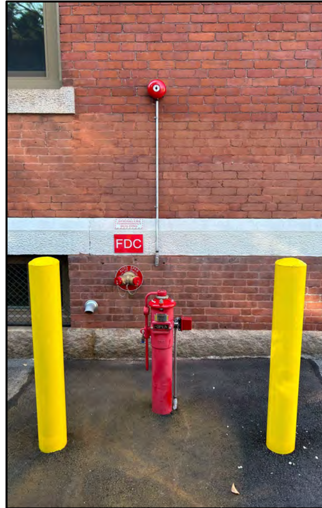
New fire sprinkler PIV
