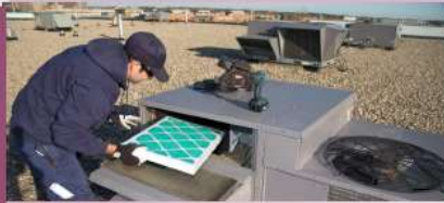
Ventilation System Maintenance
