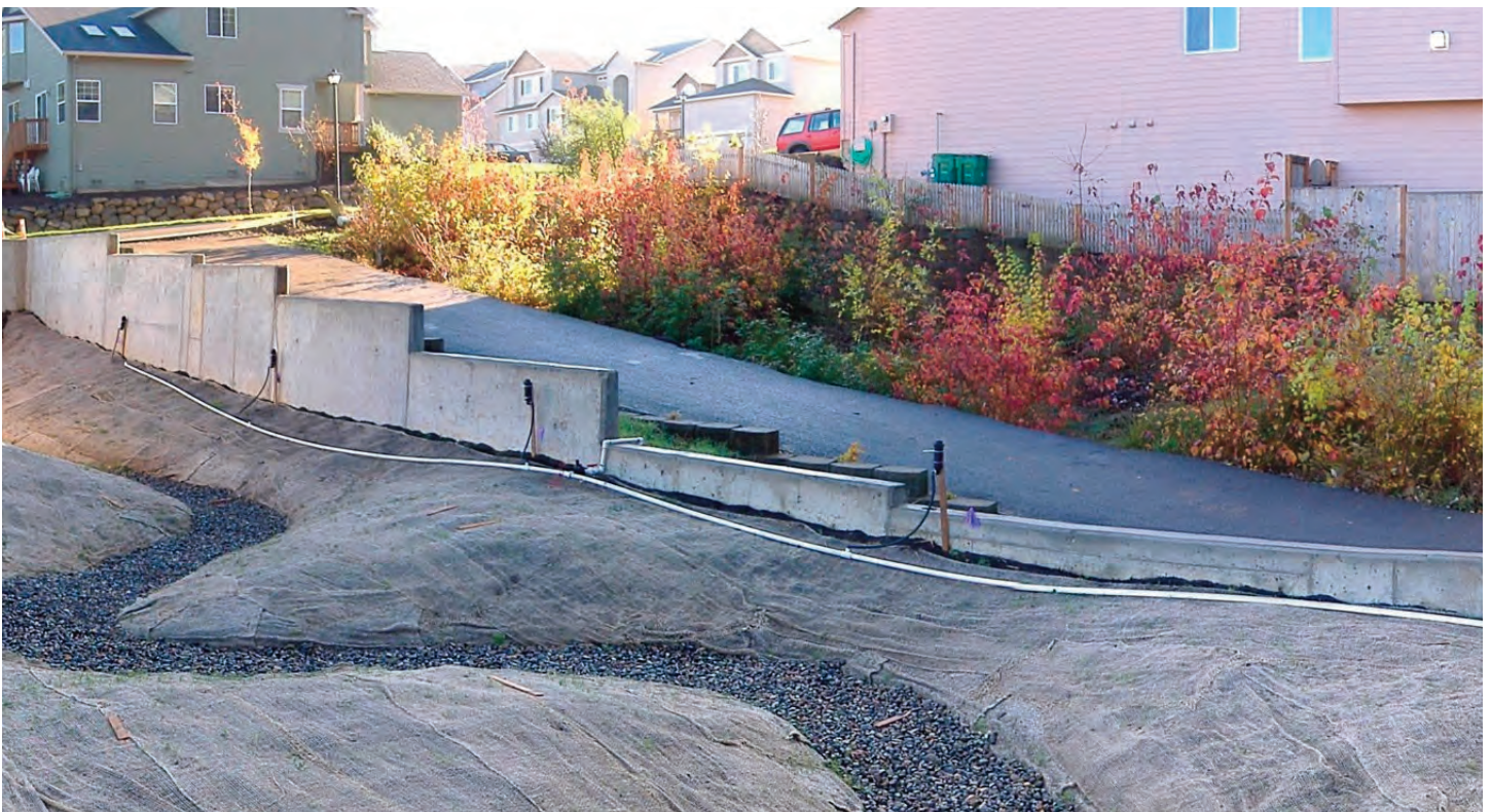
Two bioswales within a residential development: in the back, a completed planted bioswale; in the foreground construction showing water-collection area (with coarse stone) and drainage path, before soil and plants have been added.
