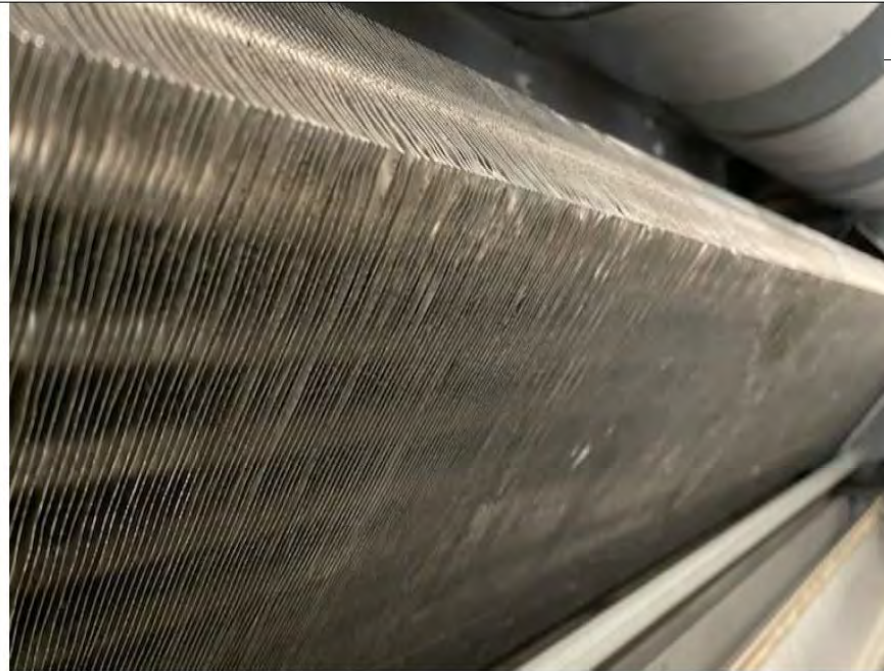
Refurbished Unit Ventilator
