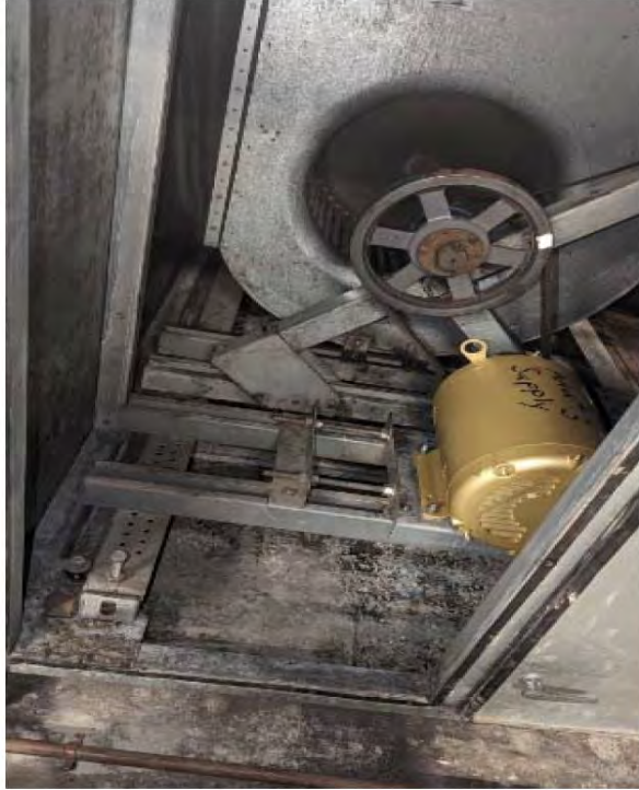
Interior of dirty AHU
