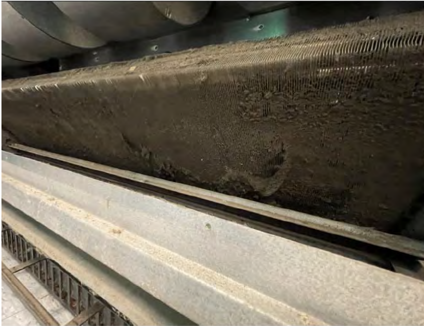
Dirty Unit Ventilator
