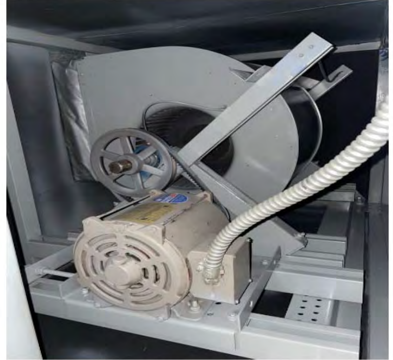
Interior of refurbished AHU
