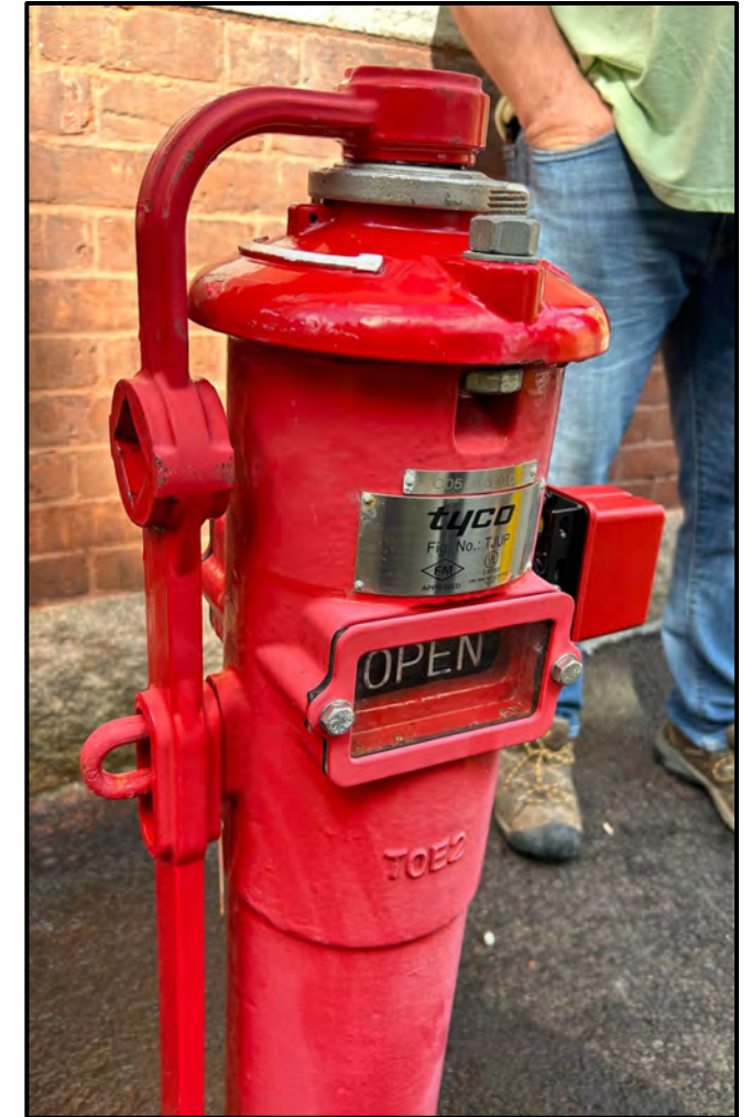
New fire sprinkler PIV (detail)
