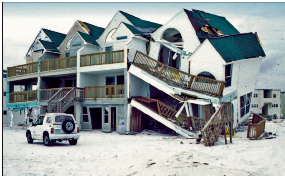
Figure 4-8. Flood and debris damage to new construction in Zone A (Hurricane Opal, 1995)
