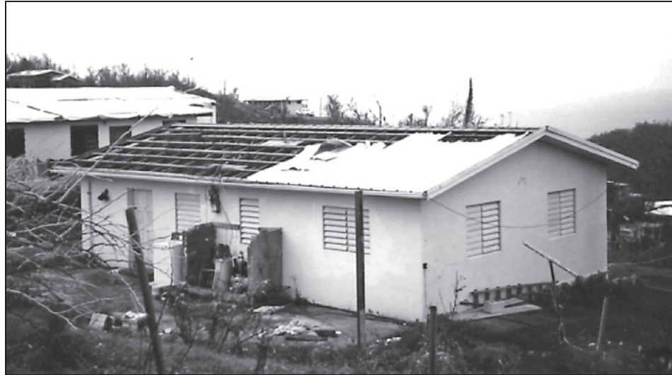
Figure 2-6. This house lost most of its metal roof covering due to high winds during Hurricane Marilyn in 1995 (location unknown) SOURCE: NRCA 1996
