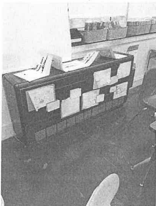
Unit ventilator (univent)
