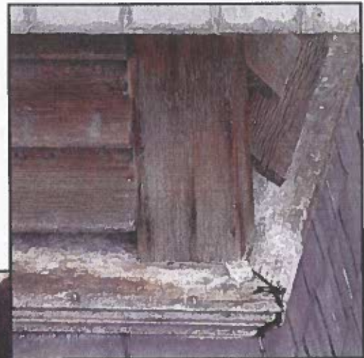
Photo 19: Detail of cupola showing gap at sill corner that was original covered with flashing, and moderate weather checking in louvers. Reflash sill corner joints. Replacement of louvers is an option, but not critical as they seem to be solid despite the weathering.
