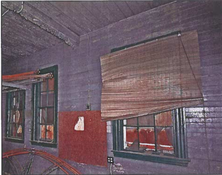
Photo 64: Interior of main barn first floor showing matched boarding on walls and ceiling that is the original interior finish and should be retained and preserved. Beam in ceiling is the bottom chord of a loft level roof truss
