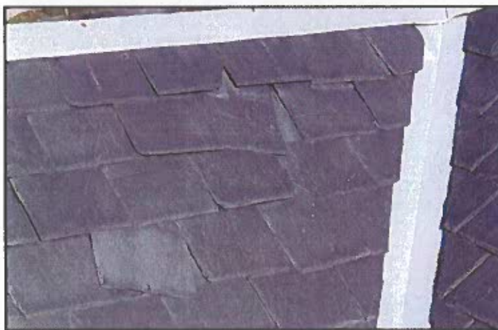
Photo 13: Slate defects - Slipped slates at top of valley shown in Photo 12 need to be refastened. This may be due to a failure of the nails to hold in the wood shingles below.
