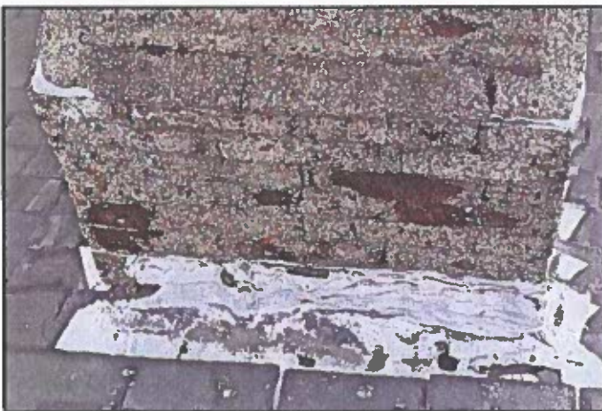
Photo 61: Chimney flashing at roof has numerous large holes that are causing leaks in the roof below.
