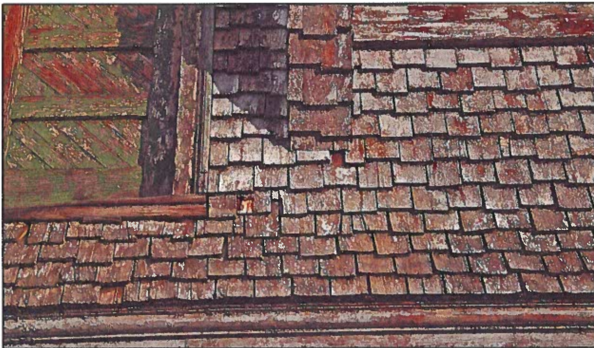
Photo 29: Shingle band adjacent to Dormer #1 on west facade showing many warped, split and missing shingles in lower portions. The extent of damaged shingles warrants complete replacement of shingles in this area, and possibly across the entire west facade.
