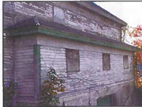
Photo 70: Overview of north ell facade showing the c. 1930s extension of the first floor. The extension does not exhibit sag of the loft wall above. However, as a precaution, the condition of sagging of the loft wall should be evaluated by a structural engineer when the basement ceiling is evaluated.
