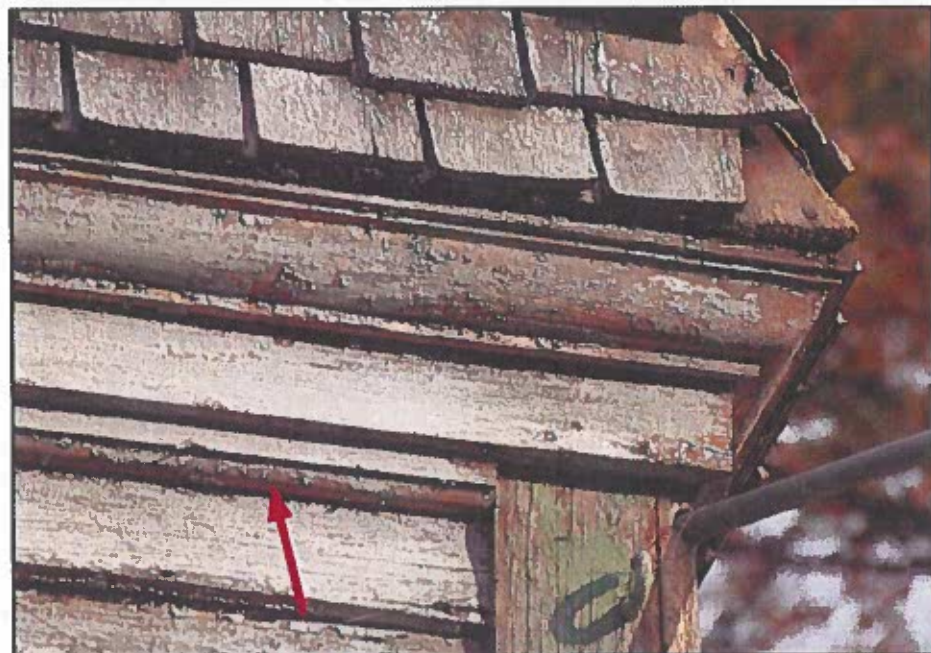
Photo 31: Detail of belt course below shingle band showing typical condition with only minor weathering. The belt course can be retained around the entire main barn (it is not present on the ell barn). However, the lowest member (arrow) and possibly other elements above it, may have to be taken off and reinstalled for proper installation of new clapboards.
