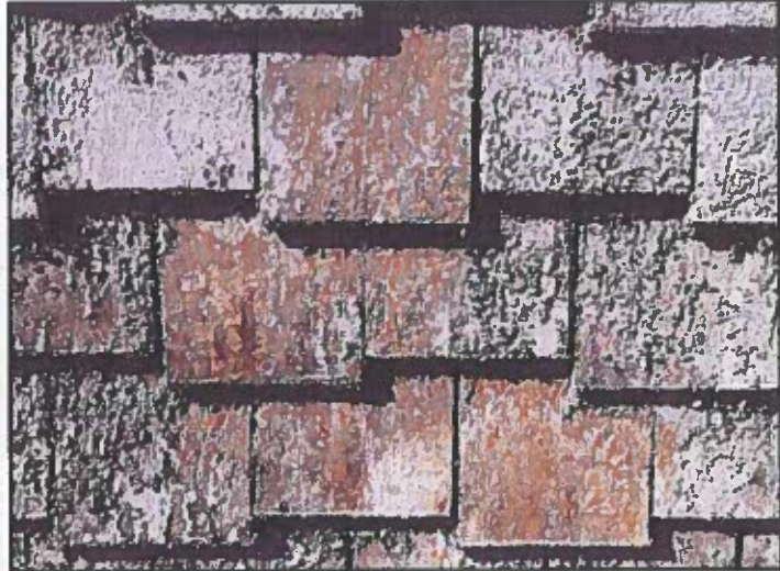
Photo 26: Wood shingles showing area where existing paint was easily scraped back to bare wood with a hand scraper. This indicate that paint to bare wood removal should be routine. The wood surface should be lightly sanded after scraping to remove surface weathering.
