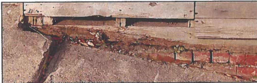
Photo 37: Sill at south facade of main barn to right of door. The face of the sill has rotted. Its condition and treatment need further investigation, similar to the sill in photo 35.
