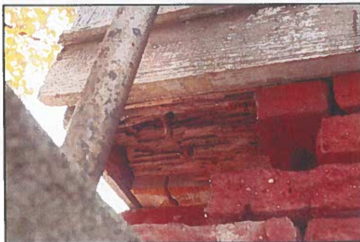
Photo 38: Sill at southeast corner of main barn. The underside of the east sill has lost several inches from insect damage and rot, while the south sill remains sound. The core of the east sill above the damage seems to be sound, and the visible damage only extends a couple of feet to the right. However, further probing should be done to verify the extent of damage. The sill needs to be repaired by piecing in sound wood to replace the deteriorated material, and the brick foundation rebuilt down to sound brick and mortar. In this case the full 12" depth of the wall need rebuilding at the top.
