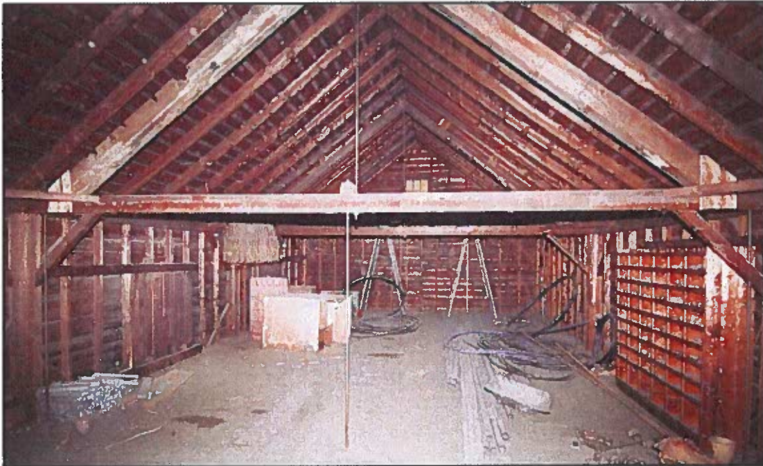
Photo 66: Interior of ell barn loft floor showing roof trusses and exposed framing. There is considerable dust and fiber debris on the floor (especially at the side walls) that is a potential fire hazard and should be vacuumed out.
