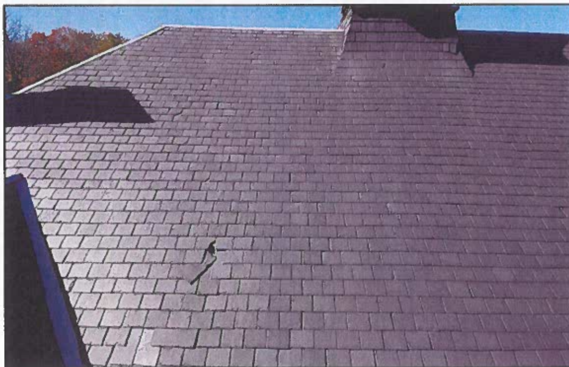
Photo 2: Southern end of east roof pitch.. Only a few slates show defects.
