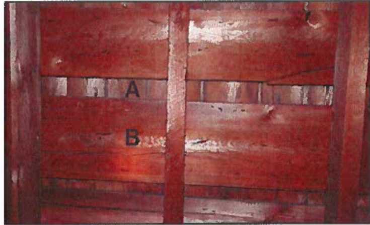
Photo 7: Underside of roof from loft showing original wood shingles (A) installed on the original spaced roof boards (B). Nails visible on underside of boarding are from shingles. Slate nailing is primarily held by wood shingles.
