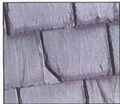
Photo 14: Slate defects - Broken corner. As break is not within 2" of joint between slates in course below, it can be left as is.
