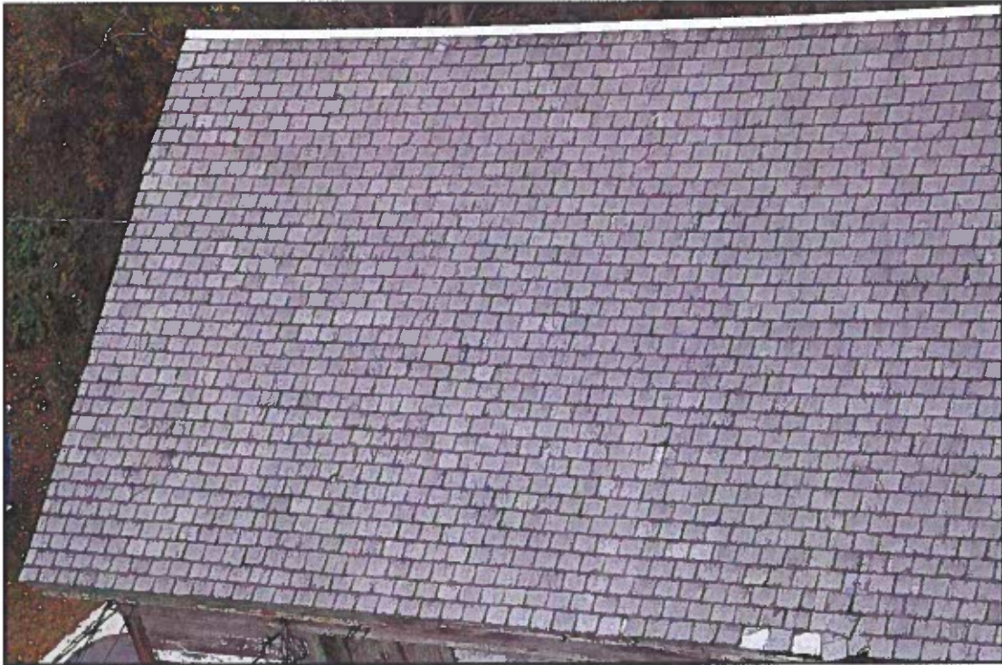
Photo 3: South pitch of ell barn roof. Note missing slates at lower right have caused considerable rot in the cornice directly below.
