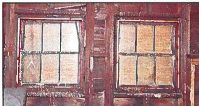
Photo 50: Interior side of loft floor main barn dormer windows showing intact sash in frames without casings. The sash and frames should be retained and preserved with reglazing unless the exterior side shows severe damage.
