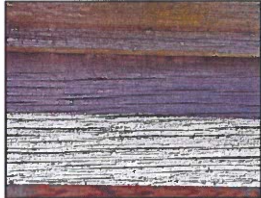
Photo 22: Detail of cornice fascia showing typical minor weather checking of otherwise sound wood. That the wood has lasted this long without rotting despite the absence of paint suggests it is more rot resistant than much modern replacement wood, and warrants retention if no other defects are present.
