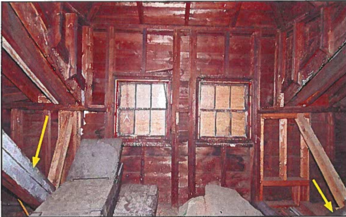
Photo 73: Interior of dormer # 4 at east wall of main barn showing past repairs to stabilize framing rotted by former roof leaks. The ends of the upper truss rafter chords (arrows) appear to be rotted completely off where they were originally joined to the floor beams forming bottom truss chords.
