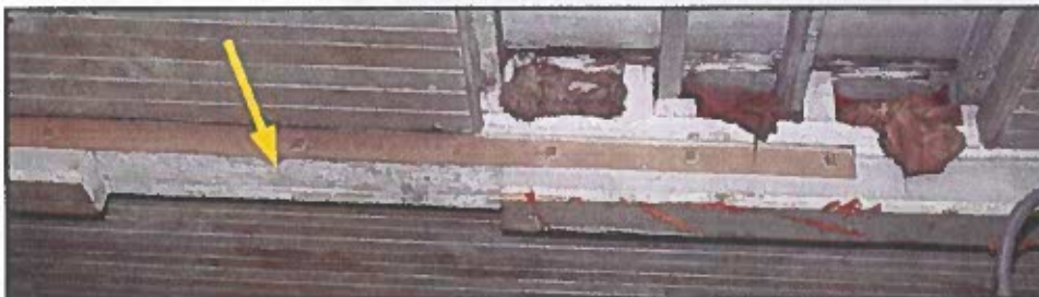
Photo 80: Bottom chord of roof truss with section cut out (arrow). The impact of this cut on the loading capacity of the loft floor should be evaluated by a structural engineer.
