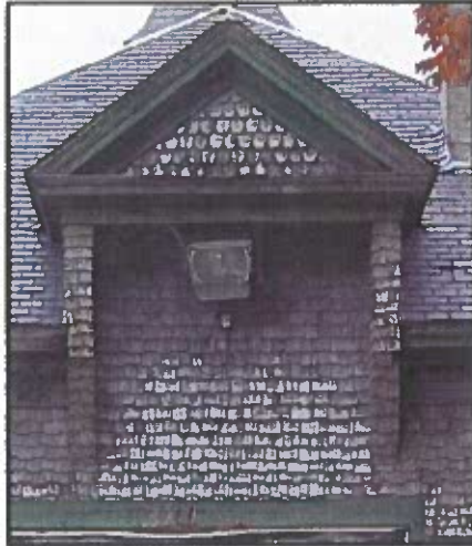
Photo 43: South facade dormer with shingled wall covering the original loft doors shown in photo 44 at right. Its original appearance matched the west facade dormer in photo 45 below.
