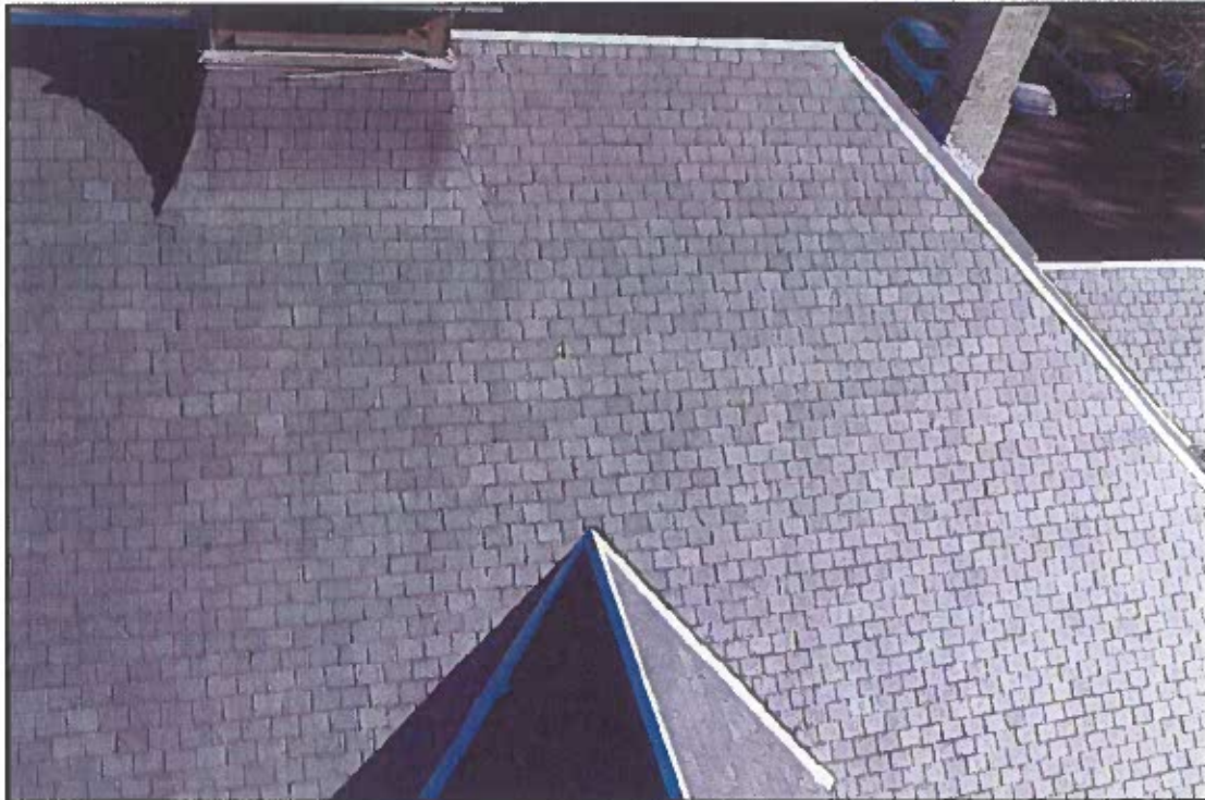
Photo 5: Southern end of west roof pitch on main barn. Only a few slates show defects.
