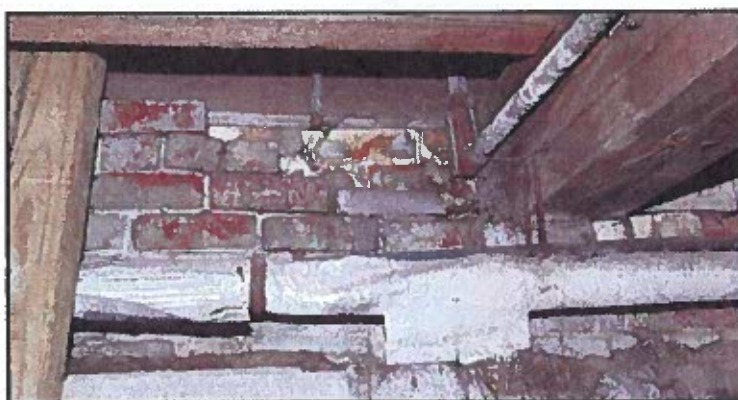
Photo 68: Basement of main barn showing obsolete steam pipe with deteriorating insulation that may contain hazardous materials. The insulation should be evaluated by a professional hazardous materials consultant and remediated as directed by the consultant.
