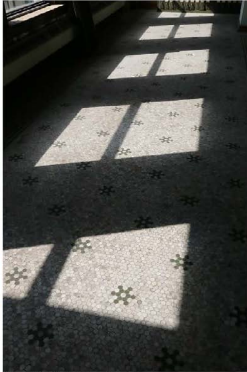
Figure 59: Tile detail on third floor.
