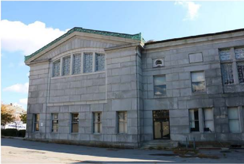
Figure 17: Rear Entrance to 1898 Building Complex. Stone Trim around Windows suggests Possibility of Additional Windows in Original Construction.
