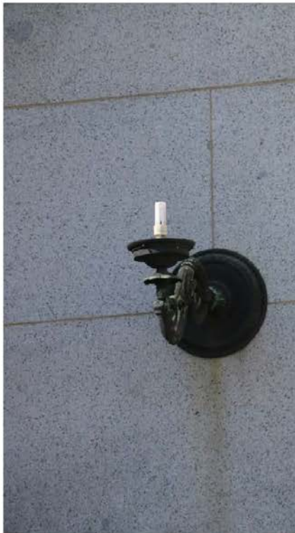
Figure 12: Ornate Wall Light (Glass Shade Missing)
