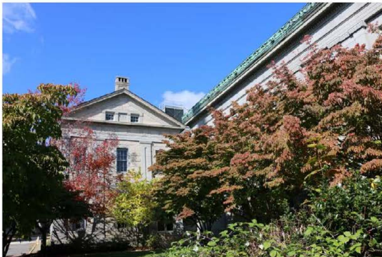
Figure 3: 1878 Addition (center) and Circa 1898 copper roof edge detail on 1845 Original Building (right)
